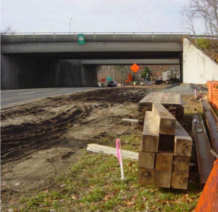
Construction stakes have been placed between sta. #15-16 in preparation for trench work. Some materials were also being stored here. Heavy rutting was observed along the shoulder with minor sediment tracking on the roadway.
