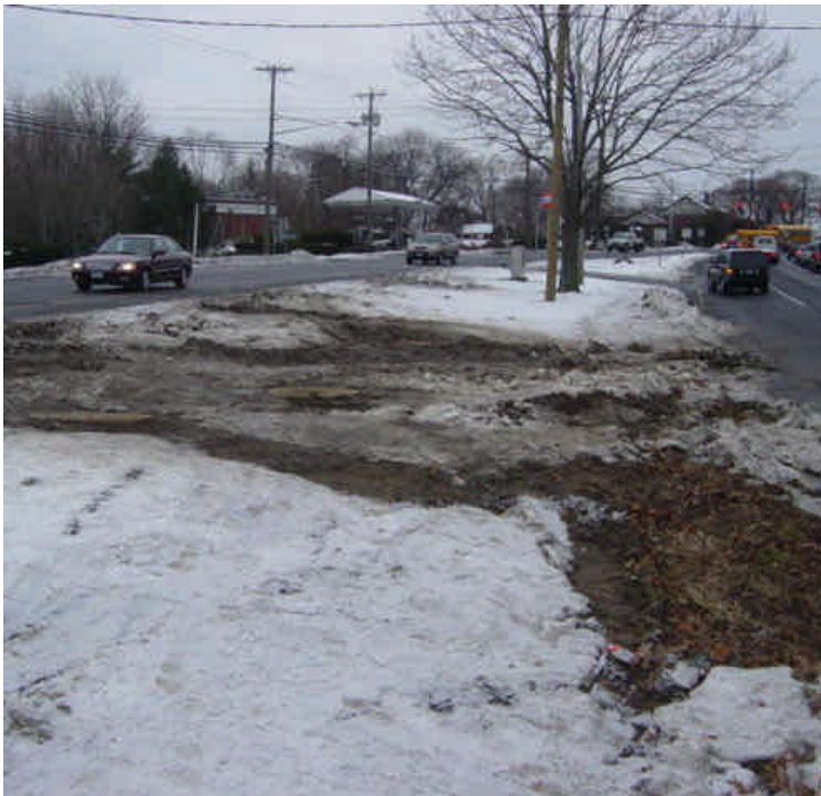
Heavy rutting continues within the median near sta. #316-318. Snow/sediment was encroaching on the roadway slightly. This area needs to be stabilized as soon as feasible.
