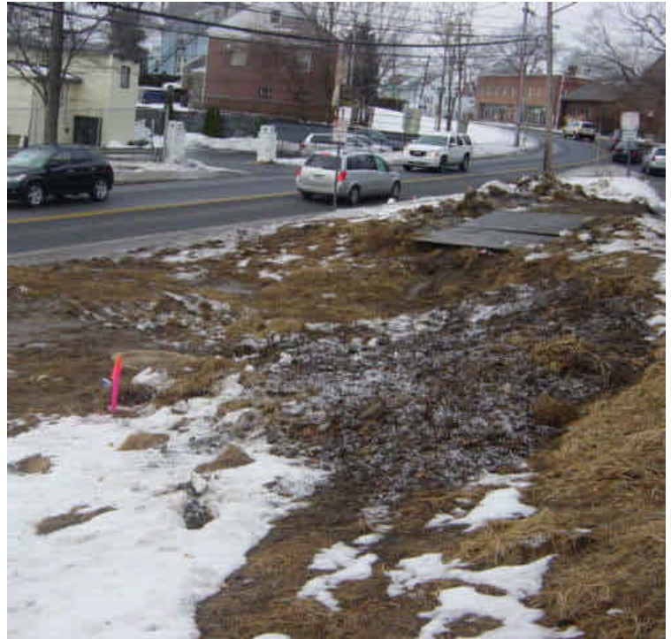
Silt fence was removed from the curb line near sta. #81 (vault #5) either due to construction or snow plowing. Exposed soils were partially mulched with hay. Continue to stabilize and sweep minor amounts of sediment along the curb.
