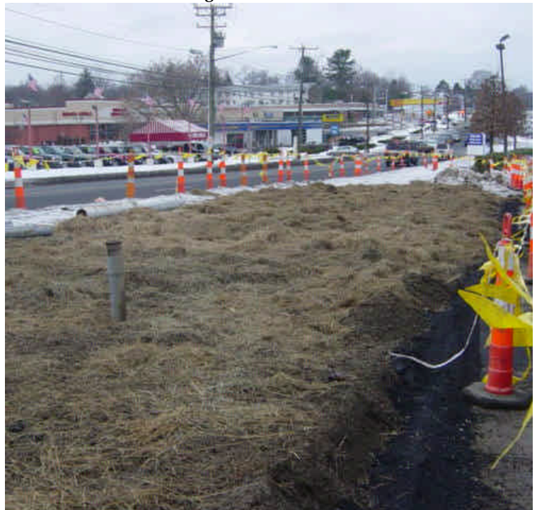
The area between #129-131 has been backfilled and mulched with hay. A temporary bituminous curb was installed but slight sedimentation had occurred within the parking lot. Sweep as needed.
