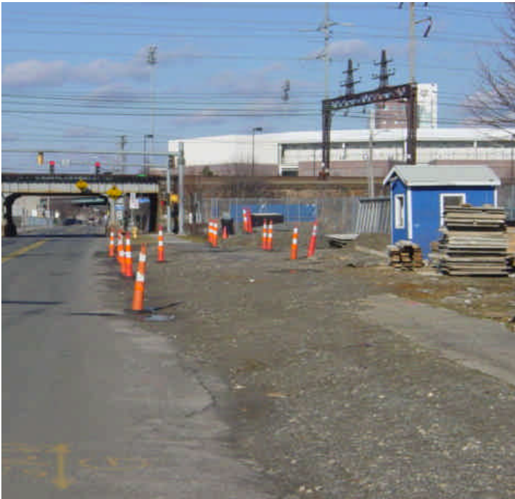
Exposed soil along the shoulder near sta. #801-803 continues to migrate into the roadway.
