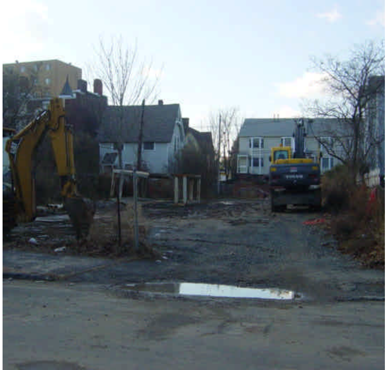
Contractors from Singer Substation project continue to store materials and equipment in the area between Broad St. and Main St. Neither tracking, nor ruts were issues here. They have stated they will be responsible for final restoration here when their access needs are complete.
