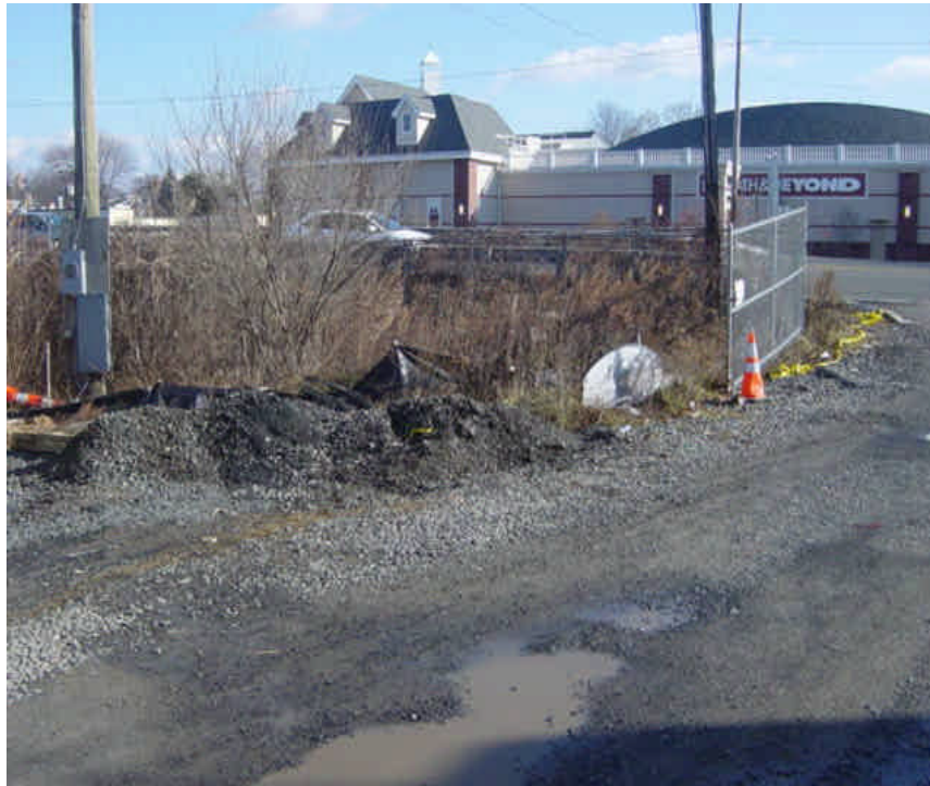
Perimeter controls remain in place around the Kings Highway laydown yard. Sediment tracking was not an issue as the work has shut down for a 2-week holiday break. Crushed stone which was previously spread throughout the yard has been plowed to the perimeter controls during snow removal activities and should be re-spread.
