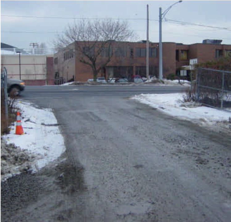
Perimeter controls remain in place around the Kings Highway lay down yard. Sediment tracking was not an issue as the work was shutting down for a 2-week holiday break.
