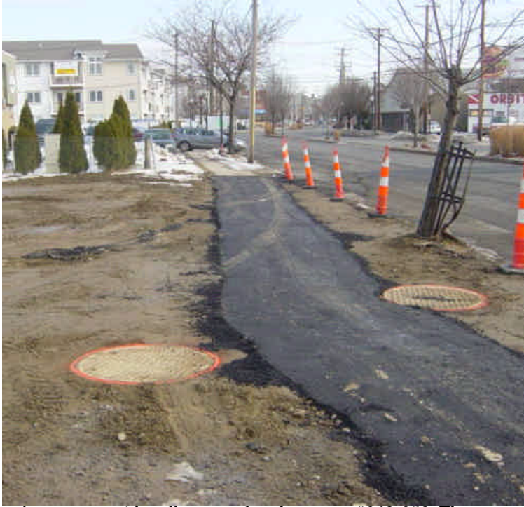
A temporary sidewalk was replaced near sta. #649-650. The adjacent lot remains exposed but some work is still needed here. The area will be stabilized when active work is complete.
