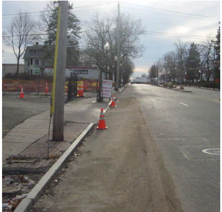
Heavy sediment accumulation was observed along the shoulders and median of Fairfield Ave. near sta. #696. The source of the sediment was apparently due to a house fire.
