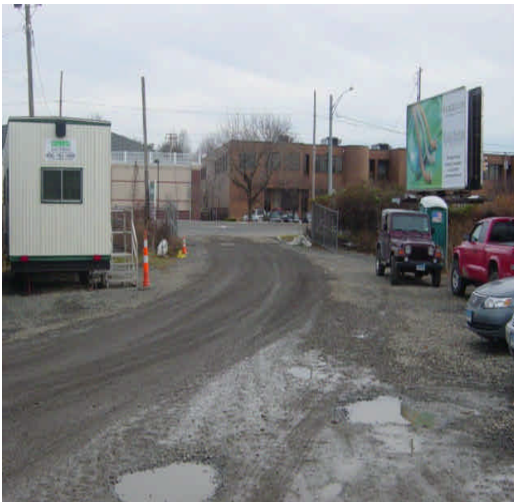
Perimeter controls remain in place around the Kings Highway lay down yard. Sediment tracking was observed. Debris material was also observed near the yard entrance.
