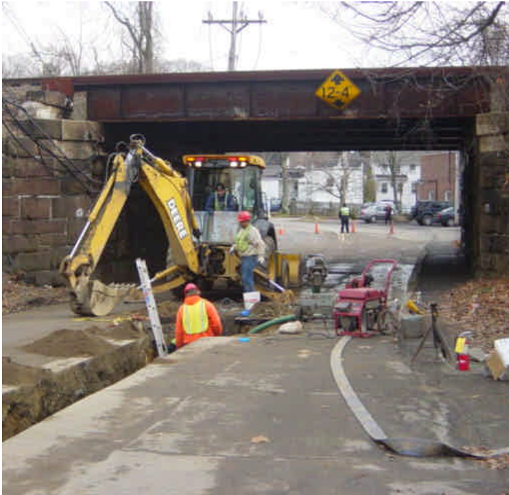
Gas main was being relocated near sta. #478-479 by Anthony Julian Railroad Construction Co. Catch basin did not appear to be protected.
