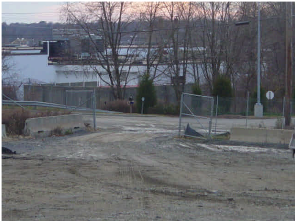
Minor tracking was observed at the entrance to the Shelland Street lay-down yard. Sweep as needed.
