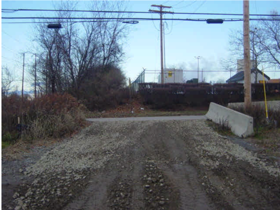
The stone has been refreshed at the construction entrance off of Caswell Street near station 1080. Overhead contractors are working in the ROW in this area.
