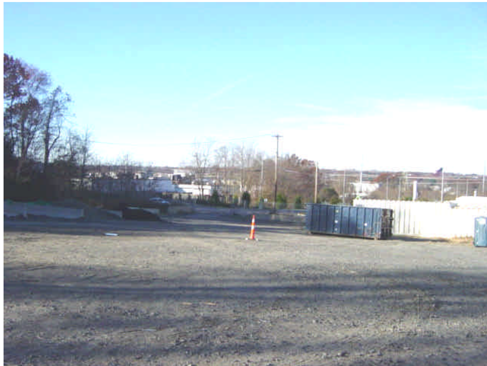
Shelland Street yard remains inactive as work has shifted to other areas of the project. Work in this segment is expected to return within the next few weeks.
