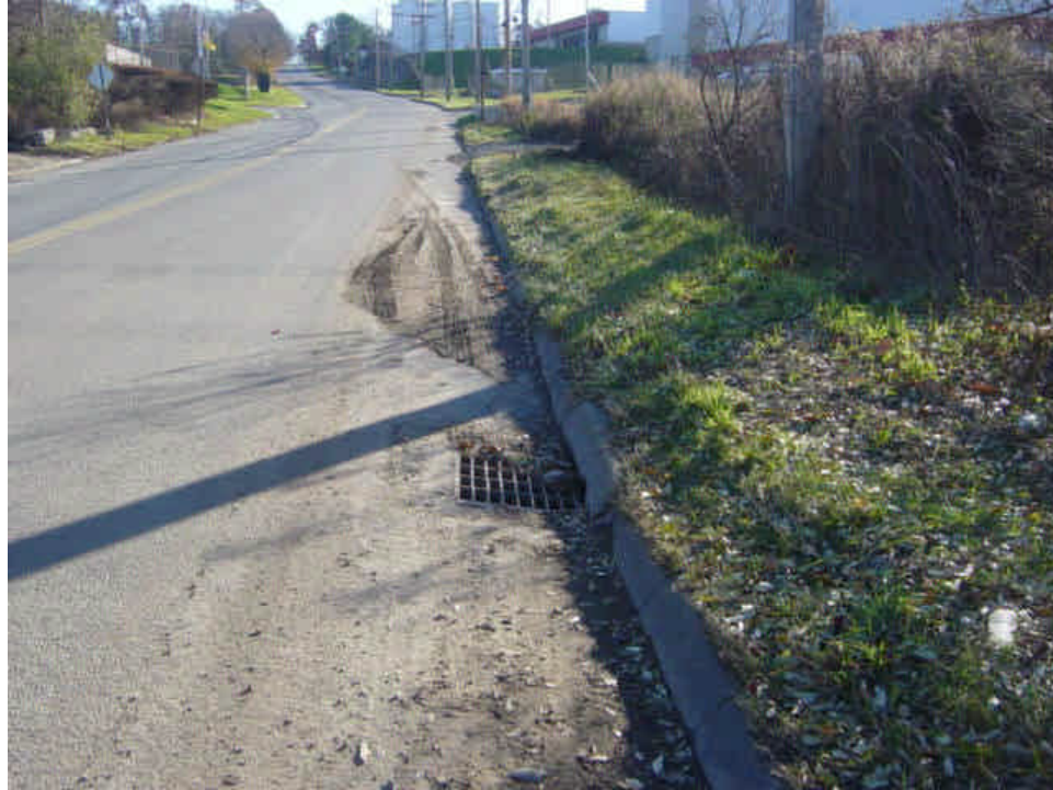
Sediment accumulation continues along Caswell Street and the catch basin is not protected. The tracking is not associated with this portion of the project. This responsibility should be coordinated with overhead contractors. See the 2B report.
