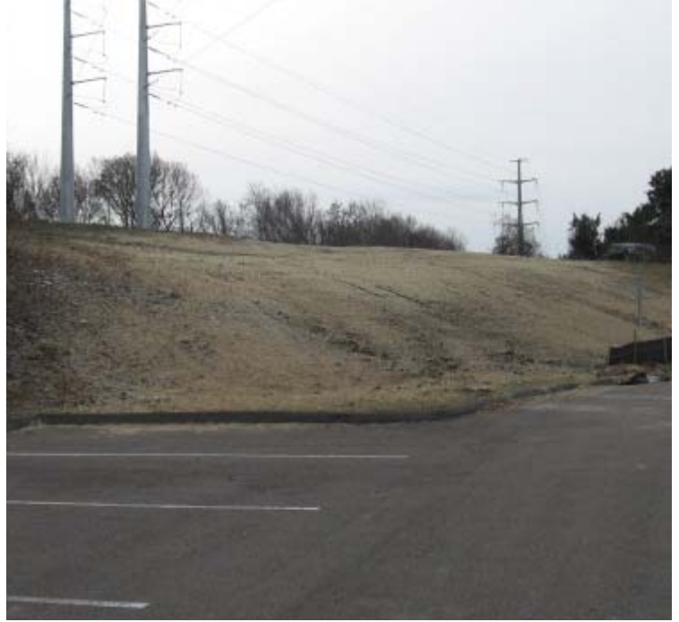
Pease Rd/JCC (Woodbridge): The ruts have been graded and exposed soils have been temporarily stabilized near structures #3931/24118. The silt fence should be extended in this area.
