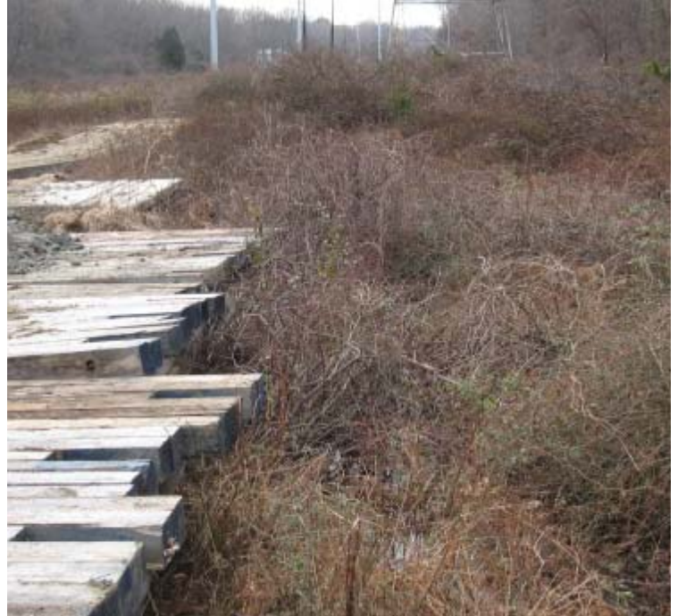
Rimmon Rd (Woodbridge): A timbermat crane pad has been installed at proposed structure #24105. The pad is adjacent/in a tributary of Race Brook. It is recommended that the work area be enclosed with erosion controls.
