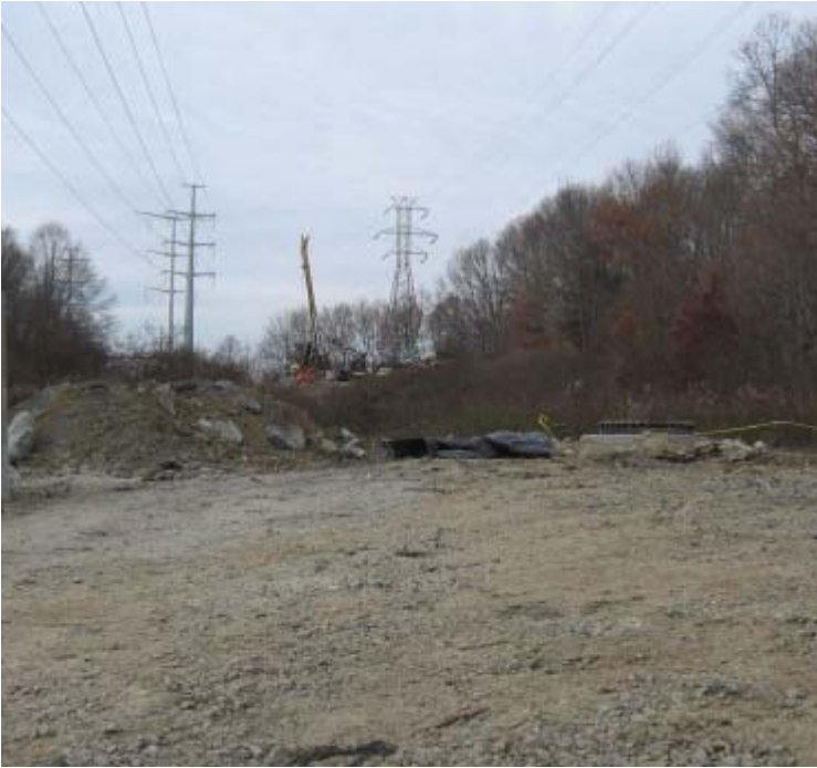
East Rutland (Milford): The foundation has been installed for Structure #24015. Spoils remain contained onsite. Foundation work continues at proposed structure #24014 (seen in the distance).
