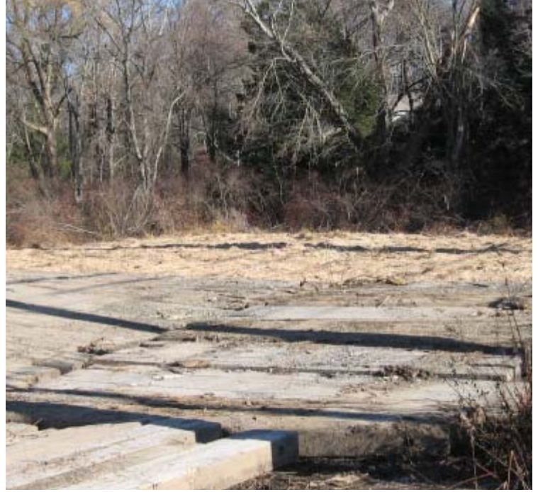
Ansonia Rd (Woodbridge): Pad reclamation is complete near structure 3914 and proposed structure 24101.
