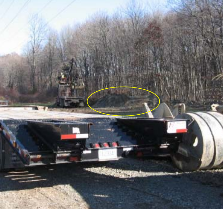
Eisenhower Park (Milford): Spoils are being removed from wetland areas and stored in the upland portions of the ROW.
