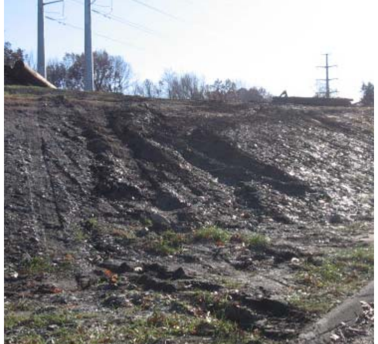
Pease Rd/JCC (Woodbridge): Ruts were observed in exposed soils near structures 3931/24118. The silt fence located at the base of the slope is in need of repair.
