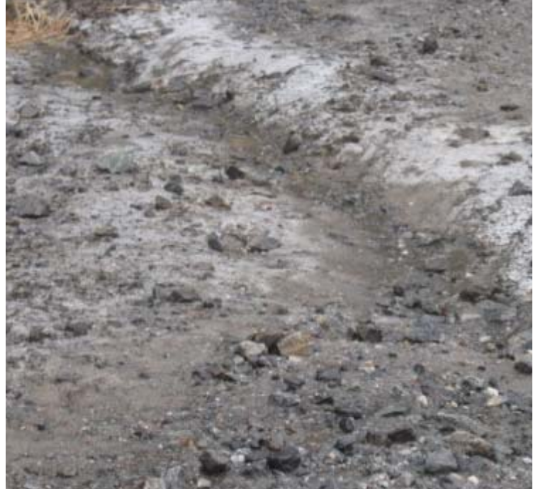
Litchfield Turnpike: An additional view of one of the recently installed water-bars.
