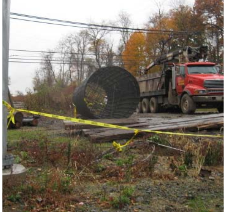
Oronoque Rd North: Spoils are being removed from wetland areas and stored in upland areas.
