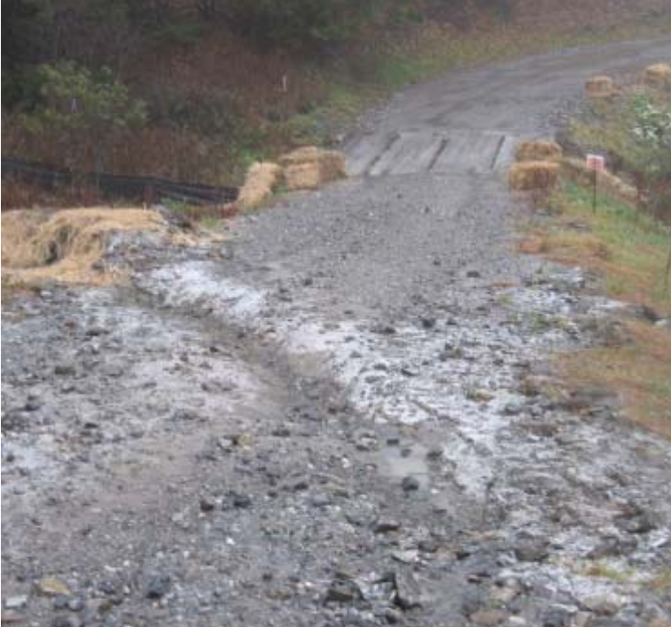
Litchfield Turnpike (Bethany): The recently installed water-bars are preventing sediment migration from the access road to the wetlands.
