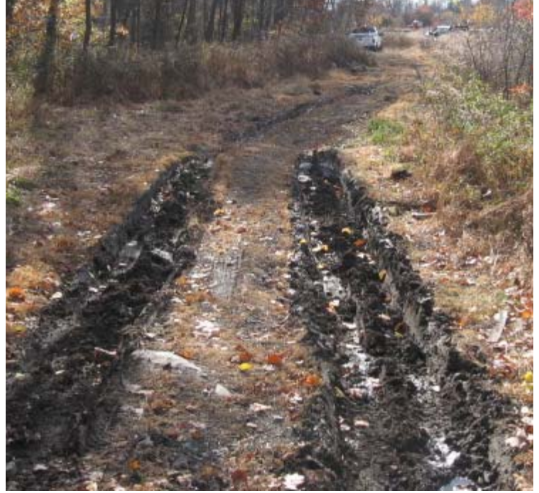
Pease Rd (Woodbridge): Tire ruts were noted within the wetland along the abandoned ROW. The vehicle seen in the distance is not parked in a wetland.
