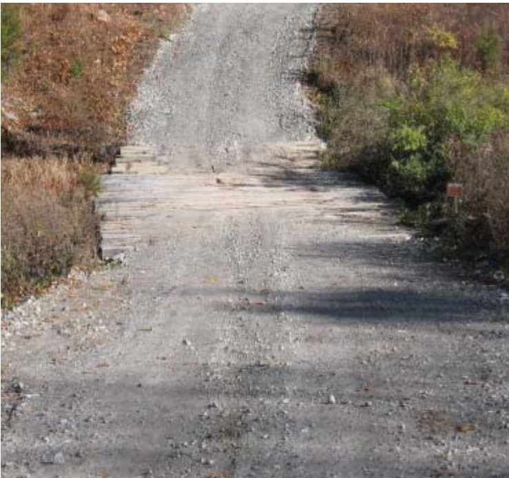
Brooksvale Ave (Hamden): Excess sediment has accumulated on the timber mat crossings within the access road at wetland #100.
