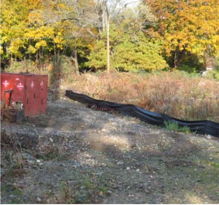
Oronoque Rd North (Milford): 345 kV foundation work is active in this area. Proper erosion controls are in place.
