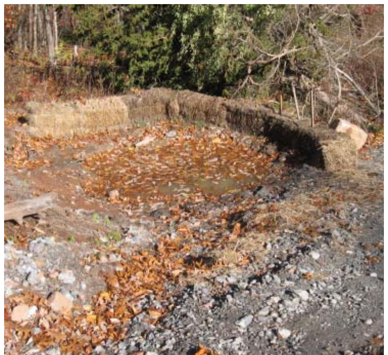
Brooksvale Ave: The haybale detention basin, located to the south of wetland #100, is functioning properly.
