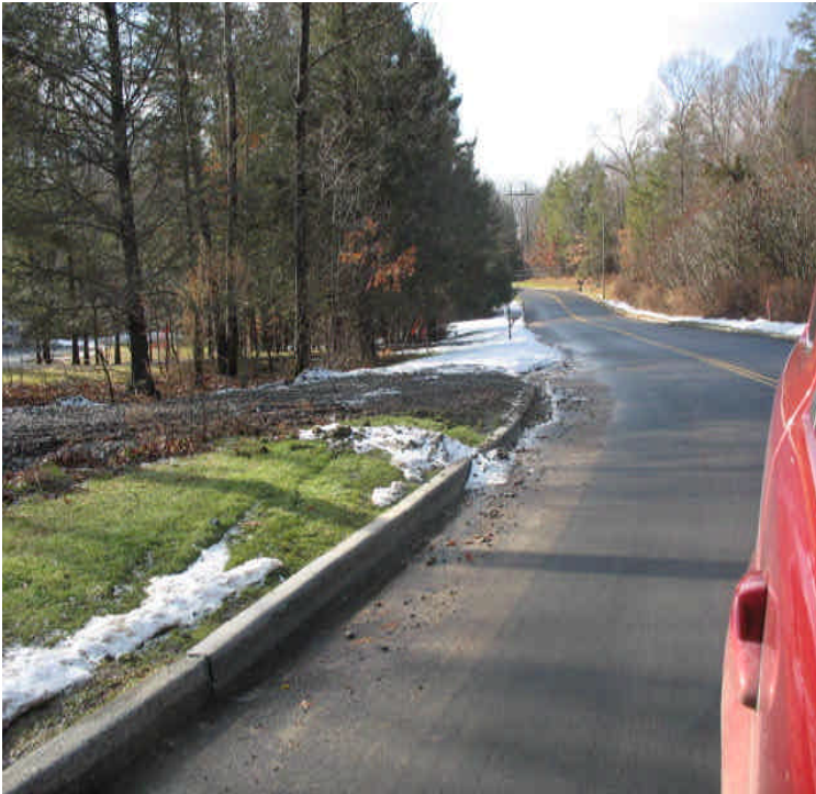
Old Farms Rd: Sediment tracking from previously active work areas.
