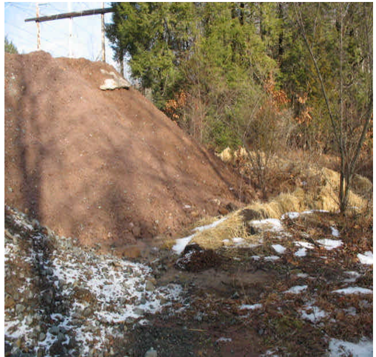
Old Farms Rd: Stockpile remains upgradient from wetlands with controls in place at its base. Remove soil when feasible as it has the potential to overwhelm the controls.
