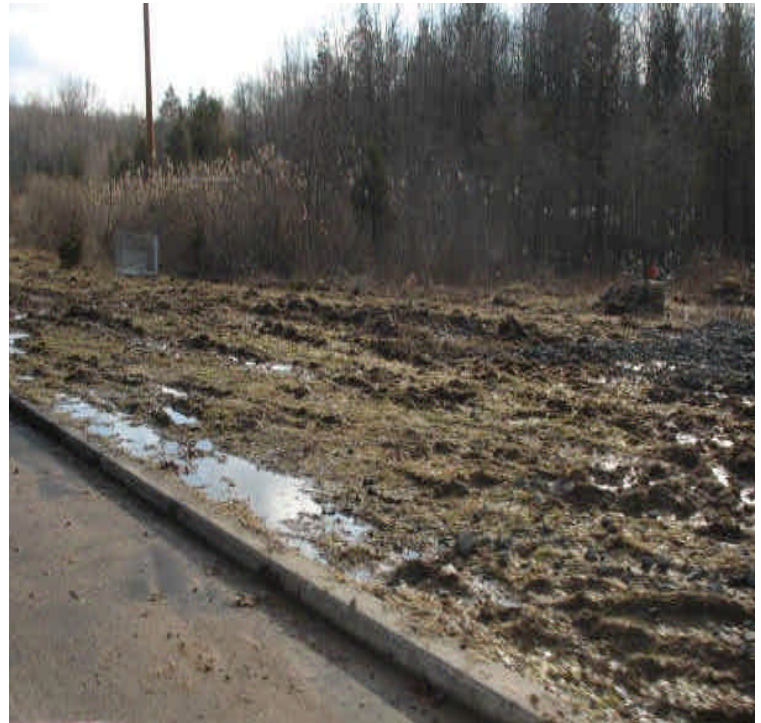
Old Farms Rd: Sediment tracking and turbid run-off noted. The previously stabilized area along the roadway shoulder was disturbed with equipment ruts.
