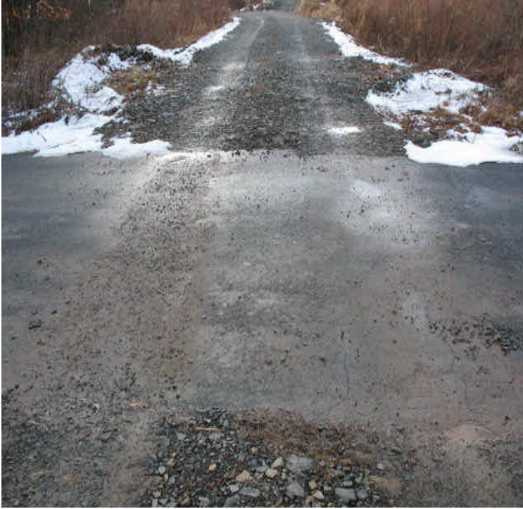
Old Farms Rd: Sediment tracking noted across private driveways.
