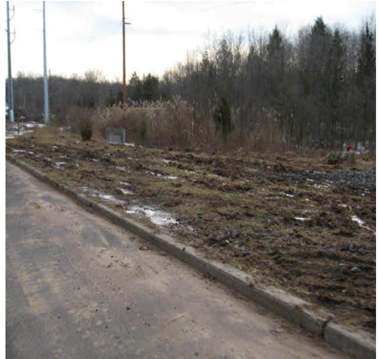
Old Farms Rd: Sediment tracking and turbid run-off noted. The area that was previously stabilized along the roadway shoulder had been disturbed and rutted from equipment. Provide additional temporary stabilization until the growing season.
