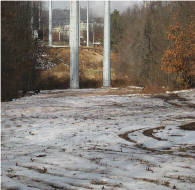
Docker Dr: Previously reclaimed areas are exposed again through ATV ruts/tracking and mulch and seed have washed away.
