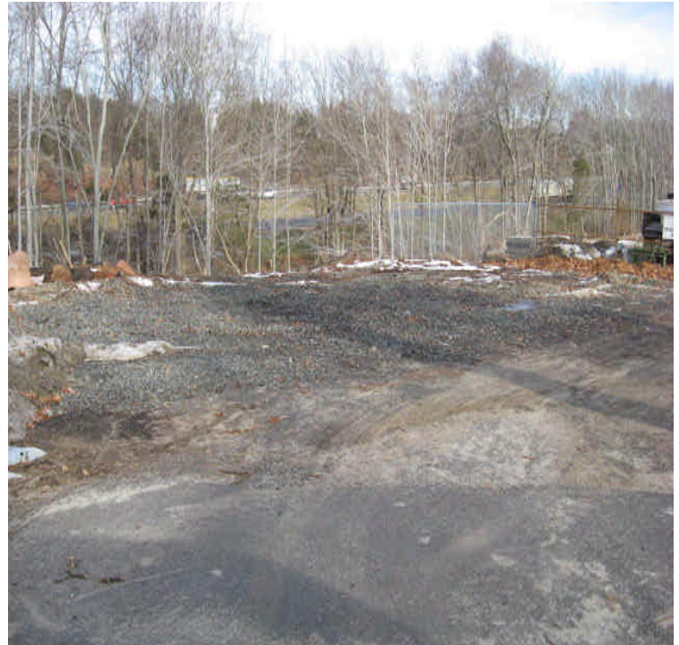
Harrison Rd.: The area where the stockpile had been removed is temporarily stable. Restore when feasible during the growing season.
