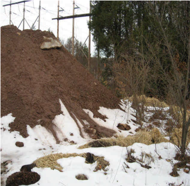
Old Farms Rd: Controls are in place at the base of the soil stockpile but the amount of soil has the potential to overwhelm them. Remove soil from this area when feasible.
