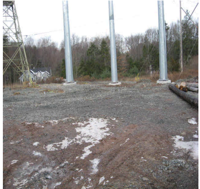
Old Farms Rd: Foundation and structures are installed. Work on temporary stabilization within approved timelines.
