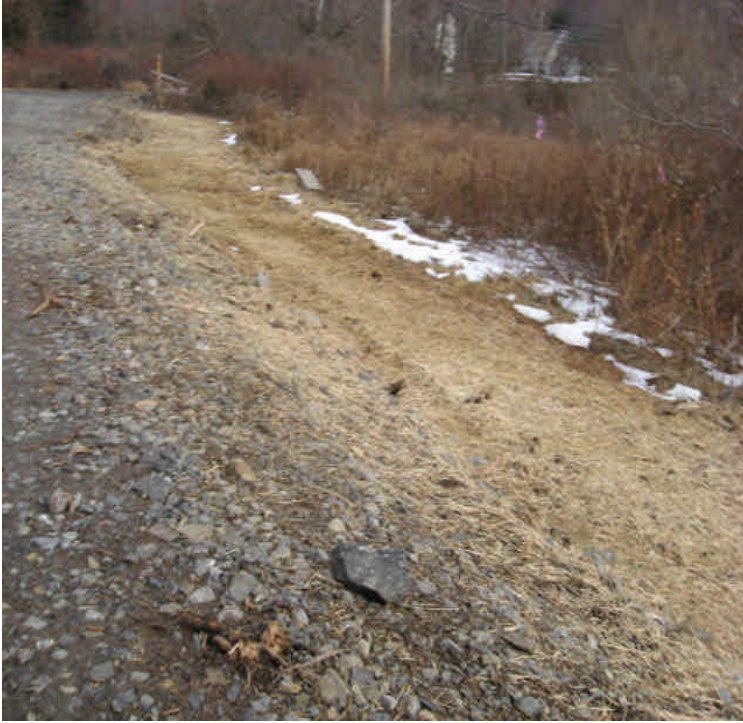
Carpenter Lane: Hay mulch and seed remain over exposed soil upgradient from the wetland.
