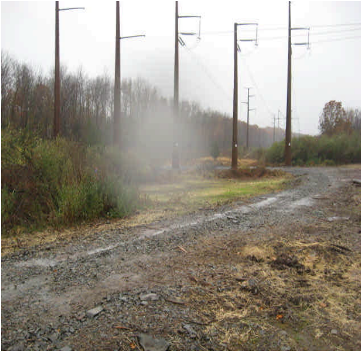
Carpenter Ln: Disturbed soils remains upgradient from wetlands. Reinforced controls are needed here.
