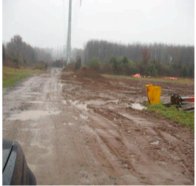
Pond Hill: The soil is being removed from the stockpile on site as it is needed. Monitor controls and stabilize disturbed soils.
