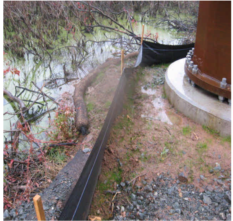
Tamarack Swamp Rd: The silt fence remains in place but the sedimen that had been pushed beyond the original controls should be removed carefully.
