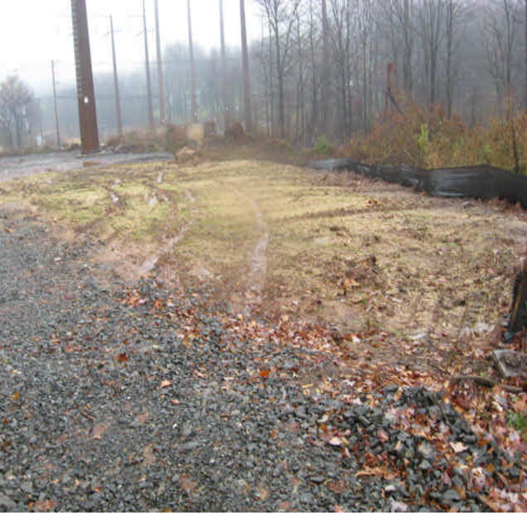
Woodhouse Ave: The disturbed area remains mulched and seeded. Minor grass growth was noted. Ensure the area is sufficiently stable for winter months.
