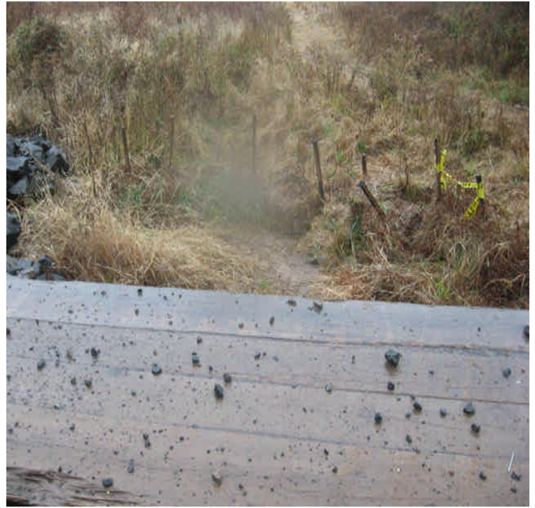
Carpenter Ln: Deteriorating controls and sediment accumulation was noted at the wetland outlet. This area still receives turbid run-off during rain events.
