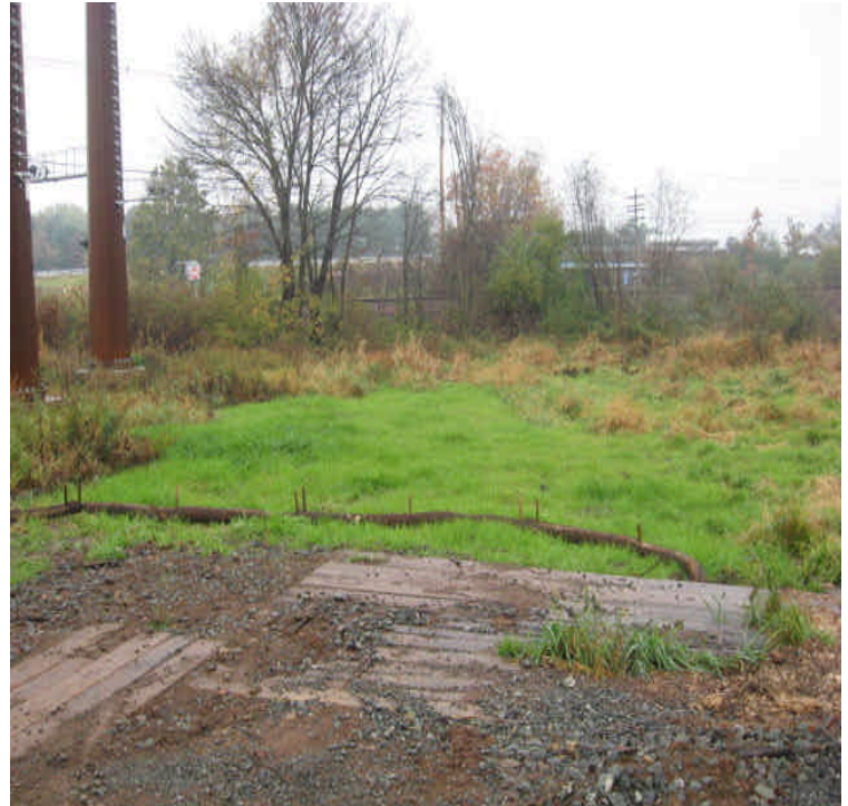
Powers Rd: The disturbed areas that were recently seeded have well-established grass cover. However, stone was not fully removed before the area was seeded and contractors are supposed to provide final restoration at this site when construction is complete.
