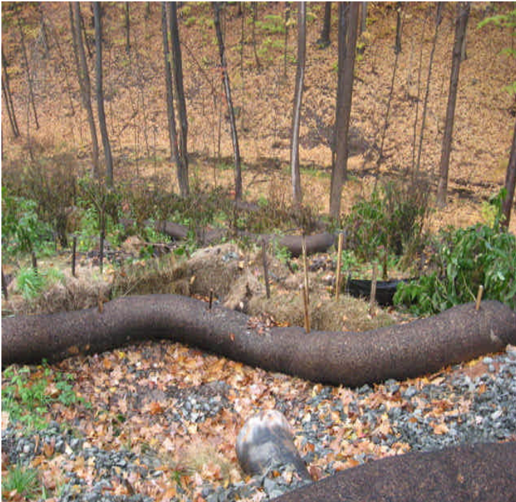
Harrison Rd: Controls at the eroded drainage ditch appear to be functioning well. However, continue to evaluate the gully and fully restore as feasible.
