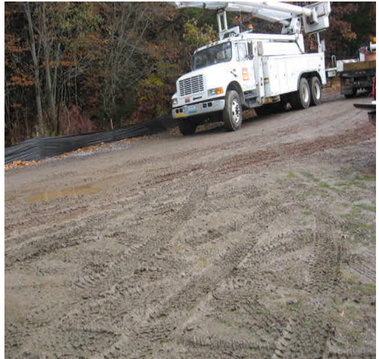
Old Farms Rd: Turbid run-off was flowing from disturbed soils on the ROW and to a catch basin in the roadway. This catch basin drains to wetlands off-site.
