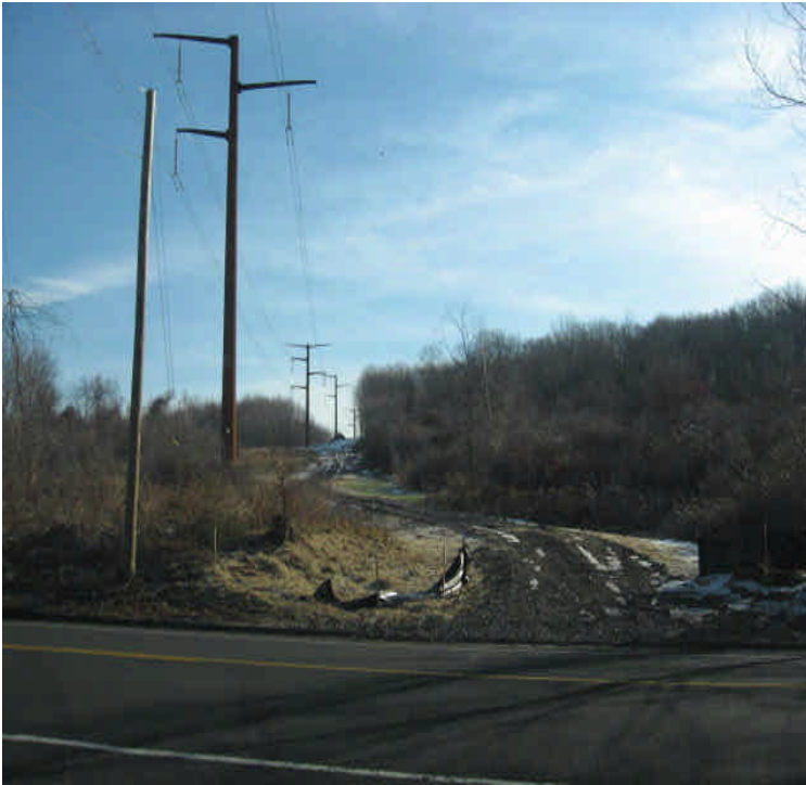
Entrance to the ROW off Rte. 17, looking to the east. Mulch and seed were in place in previously disturbed areas.
