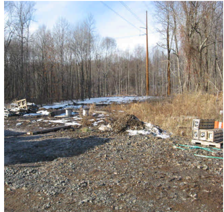
View of the turn in the ROW towards Little Lane. Controls are in place upgradient from wetlands.
