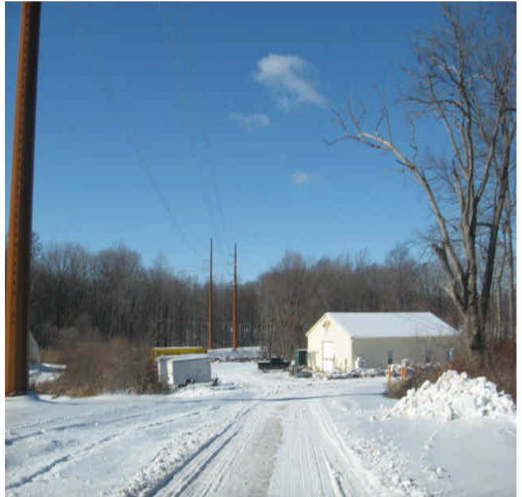
Entrance off Rte. 17, looking west into the contractor yard. The yard is starting to be demolished.
