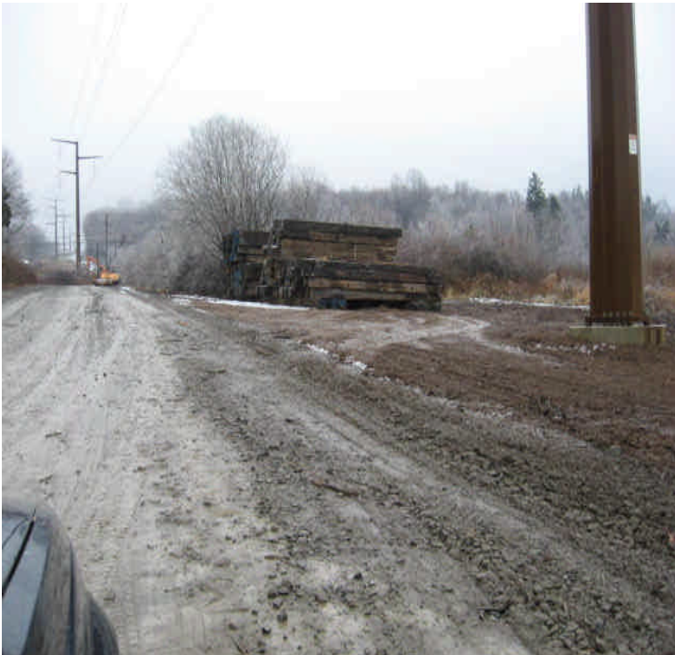
Turbid water noted flowing along the access drives within the receiving yard.
