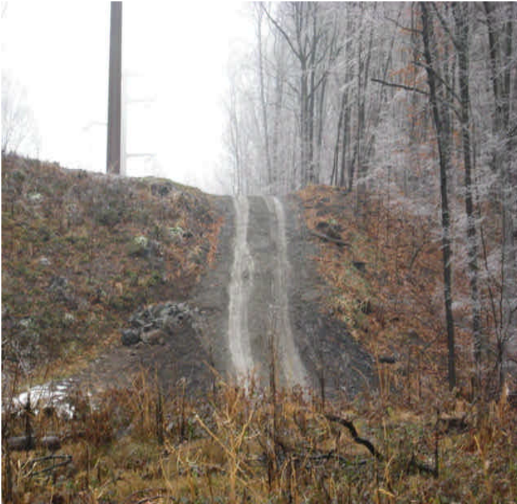
Minor erosion was no longer noted along the access road off Black Walnut Drive since the repairs had been made.
