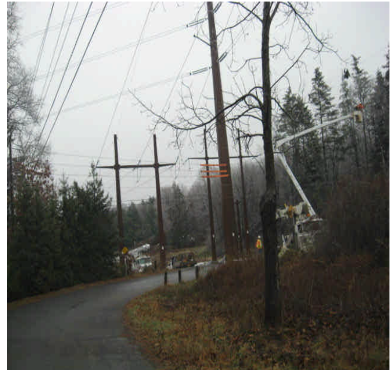
View of the intersection of segments 1A & 1B off Little Lane. Line pulling work was underway.
