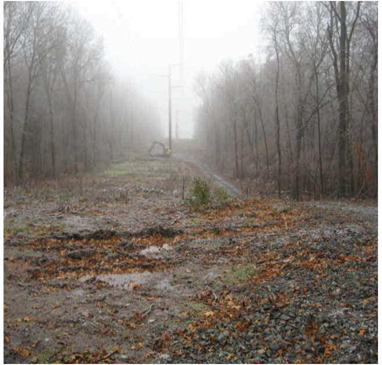
Pad work was noted at the last structure access off Black Walnut Drive
