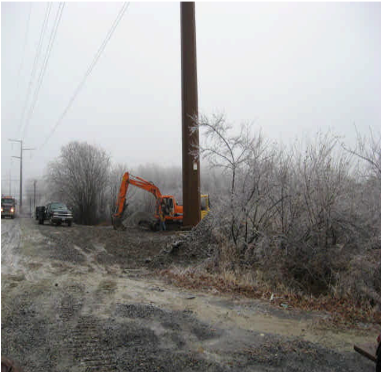
Grading and application of new stone was noted within the receiving yard. Turbid water noted flowing within the site.
