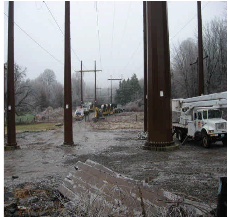
View of the intersection of segments 1A & 1B off Little Lane. Line pulling equipment was on site.
