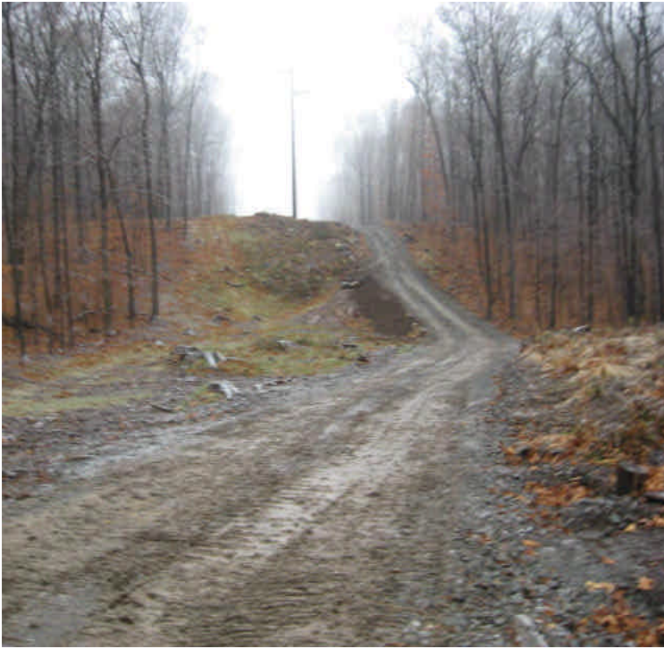
The minor erosion along the access road off Black Walnut Drive has been regraded and a water bar has been installed.
