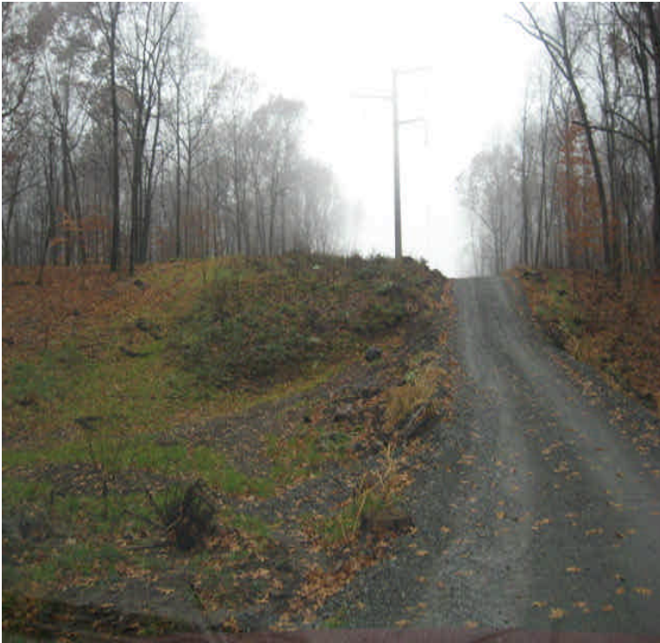
Minor erosion remains along the access road off Black Walnut Drive.
