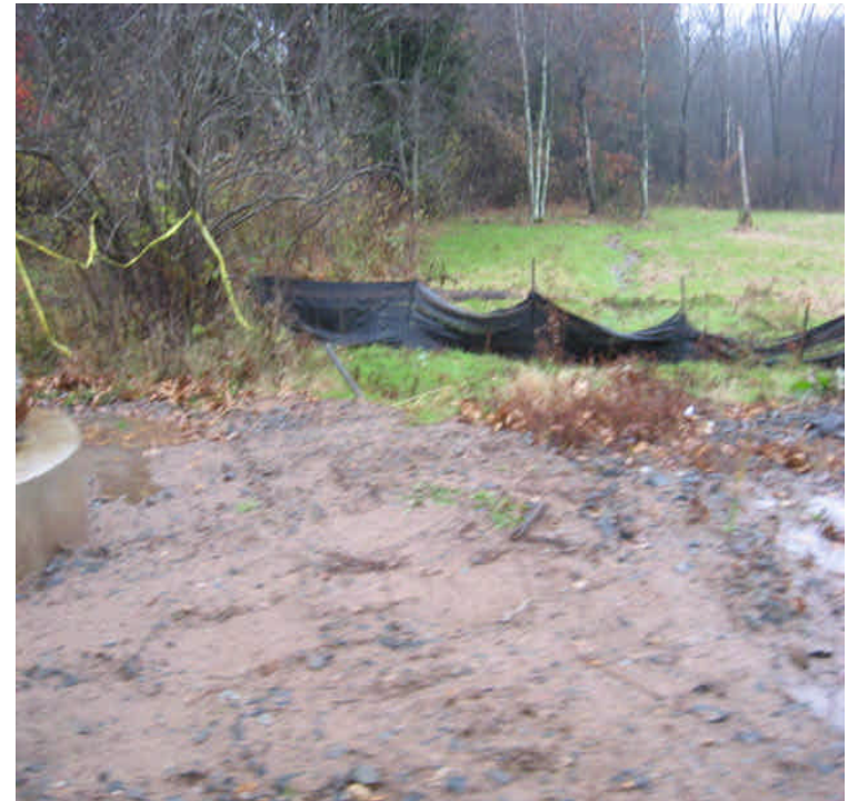
View of silt fence adjacent to wetlands at the 1A & 1B connection off Little Lane.
