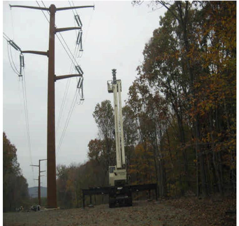
Equipment was active at the edge of the wetlands within the Laurel Brook Watershed Protection Area for line work.
