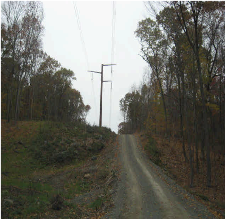
Minor erosion noted along the access road at the steep slope off Black Walnut Drive.
