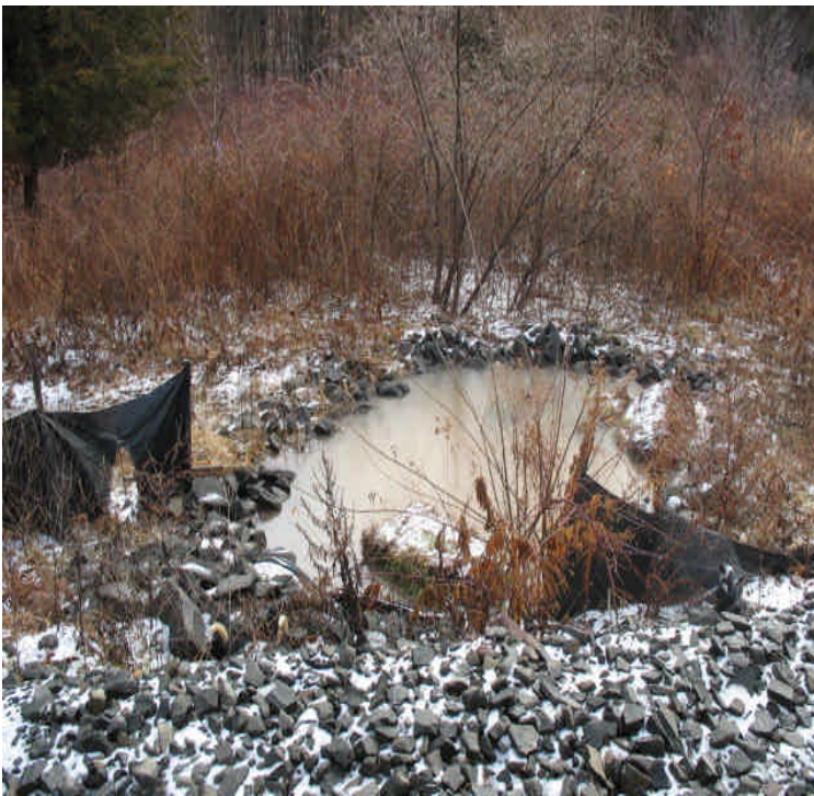
Carpenter Ln: Turbid water from access road run-off was noted in the sediment trap adjacent to Beseck.
