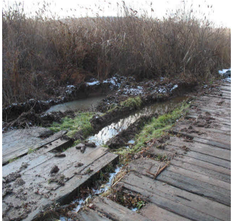
Durham Rd: View of the ruts created off the edge of the timber mats in the wetlands. This occurred several weeks ago when equipment was anchoring lines. Once crews return from break, this should be carefully repaired.
