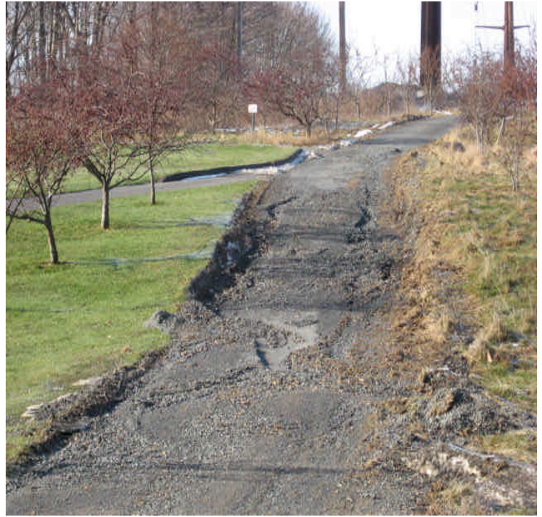
Durham Rd: Minor erosion noted along a slope on the access road.
