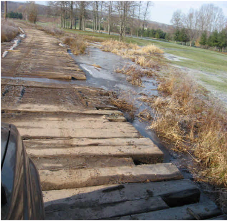
Durham Rd: Timber mats are compressing into soils at the wetland crossing
