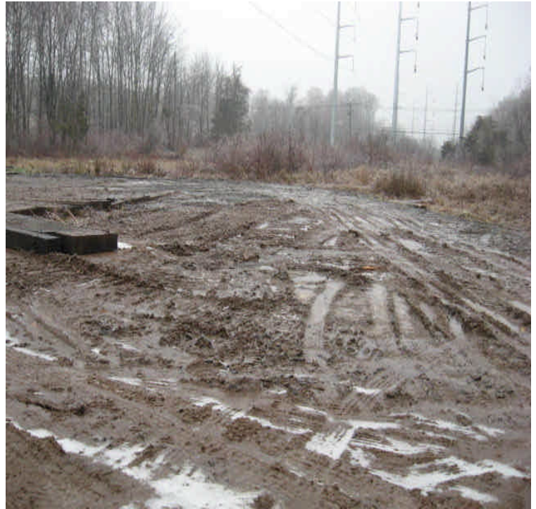
S. of High Hill Rd: Large disturbed area with mats remains partially covered with sediment. Add controls and provide temporary stabilization.
