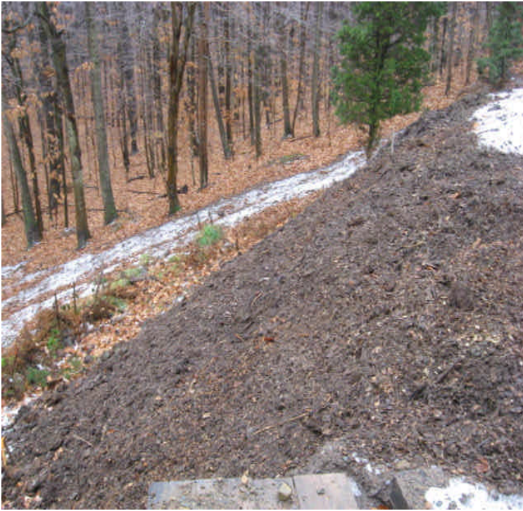
Black Walnut Dr: Silt fence remains in place upgradient from Ball Brook. The washouts on the slope have been graded and stabilized with heavy mulch.
