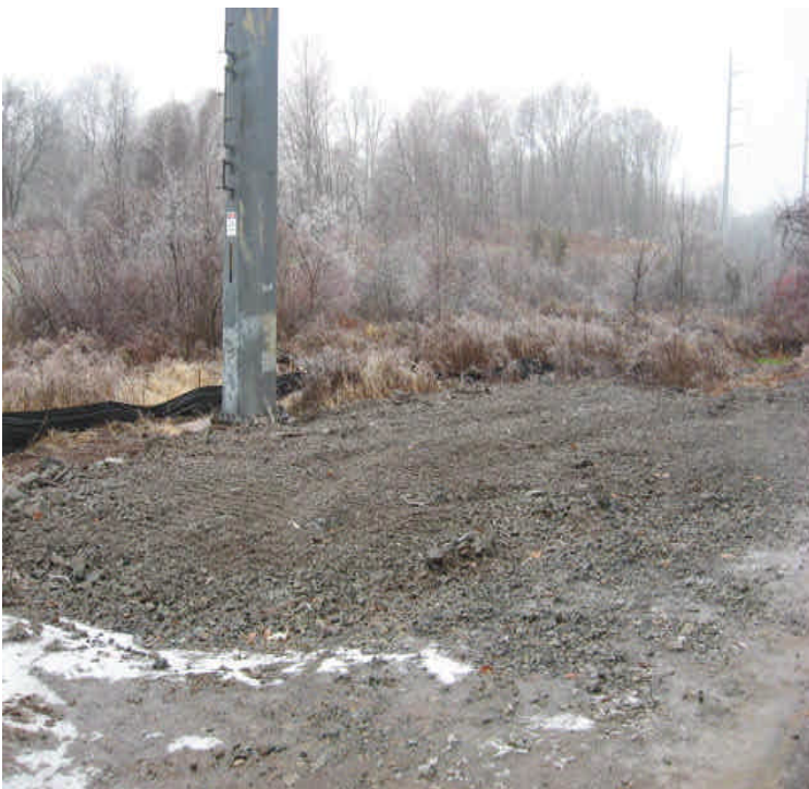
N. of High Hill: Soil stockpiles that were noted in the wetland last week were actually intended to create a lay down area for the existing structure here. Controls have been installed. Ensure all gravel is removed from the wetlands when work is completed. Timber mats may have been a better option in this case.
