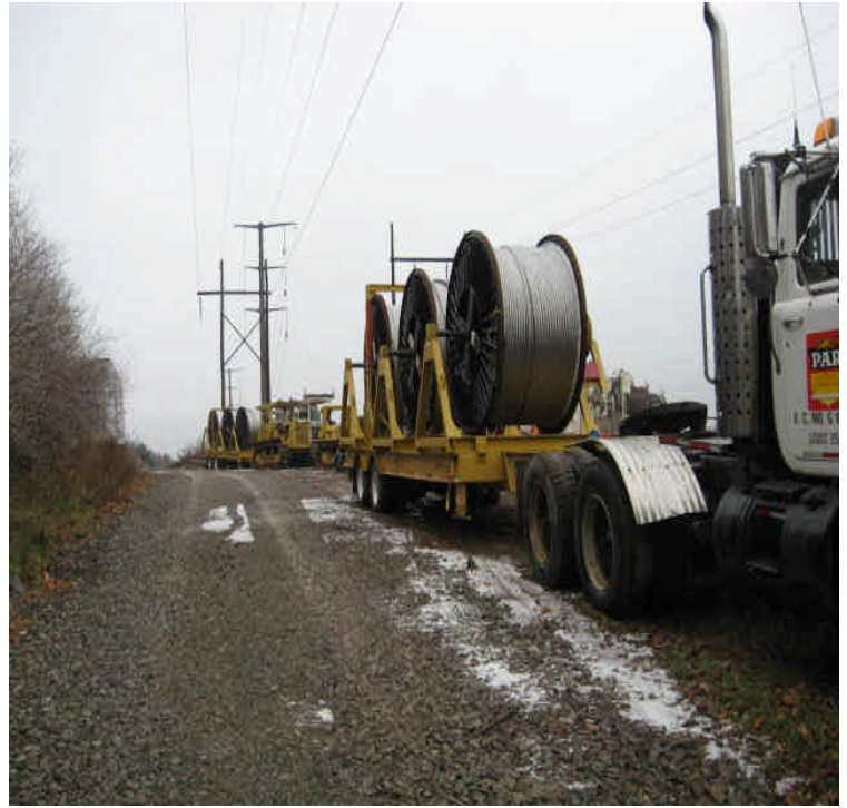
Little Lane: Line pulling equipment and crews working from Little Lane through to Powder Hill Rd.
