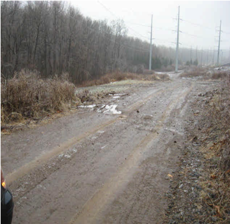
East of BSS: Drainage channels/waterbars installed to divert stormwater. Additional controls may be needed to filter stormwater before flowing off site.
