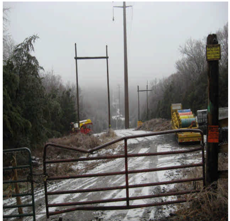
Powder Hill: Pulling equipment was in place for stringing line from Little Lane.
