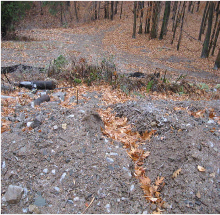
Black Walnut Dr: Silt fence remains in place upgradient from Ball Brook at the base of the washouts. Monitor silt fence but address the problem at the source. Repair the gullies and re-stabilize the slope, especially as work activities are not returning
