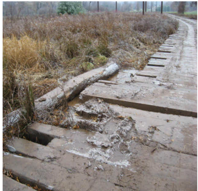
Durham Rd Golf Course: Matted access road with sediment accumulation due to timber mats compressing into the soil surface. Turbid water was noted in wetlands when mats are in use.
