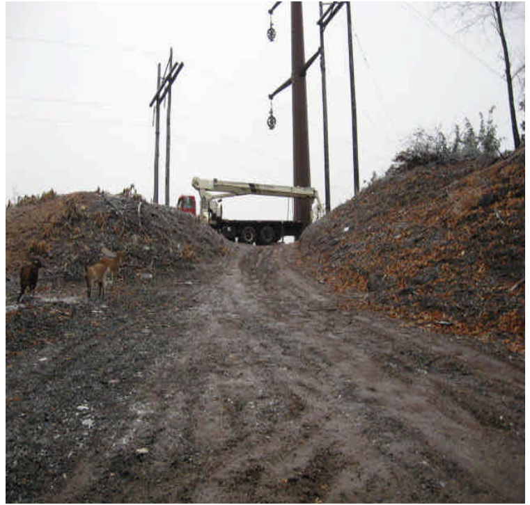
Transfer Station: Equipment was in place, preparing for line work from Little Lane through the golf course.
