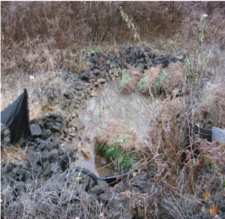
E. of Beseck SS: Turbid water from the access road was overflowing out of the sediment trap. Wetlands are located to the east.
