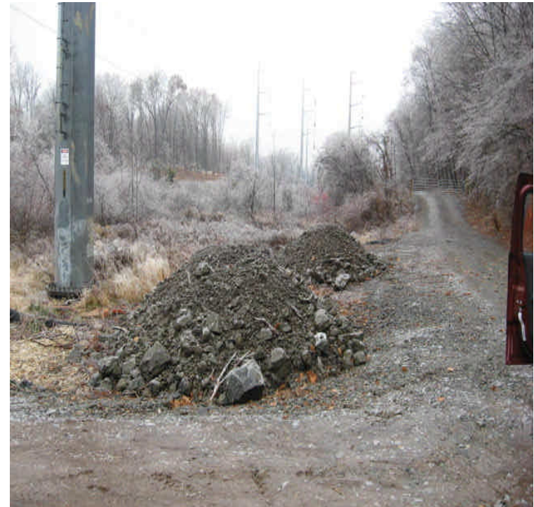
North of High Hill Rd: Three soil stockpiles were located within the wetlands adjacent to the access road and timber mat pad. These should be removed immediately. Reinforce controls to identify wetland boundaries.
