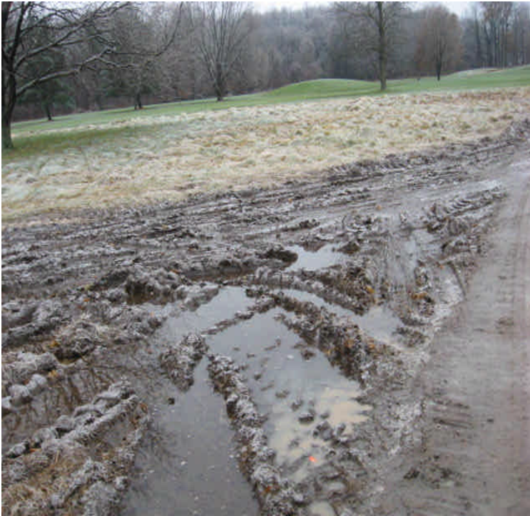
Durham Rd Golf Course: Heavy ruts from equipment were noted just off the timber mats and stone access road. Additional mats should be used here or the area should be regraded and stabilized.
