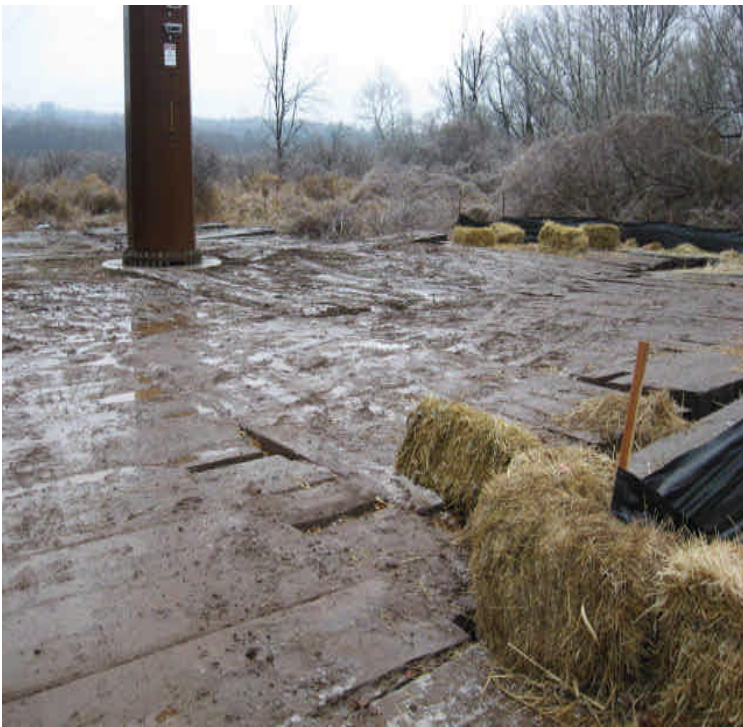
Durham Rd Golf Course: View of the structure installed within the wetlands upgradient from Durham Meadows.
