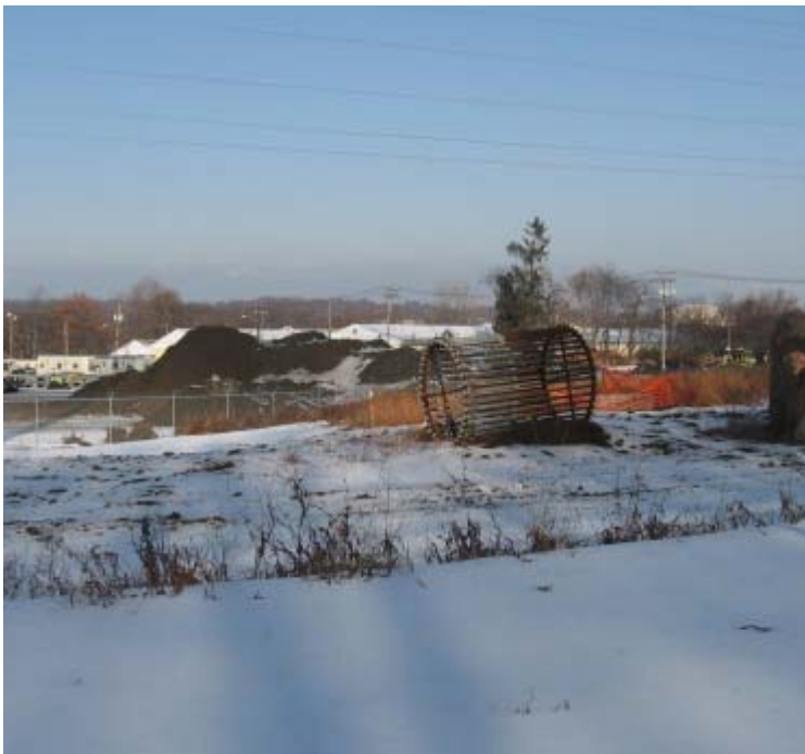
East Devon Substation: All spoils from foundation work are being stored in the northeast corner of the site. The spoils appear to be contained on site.
