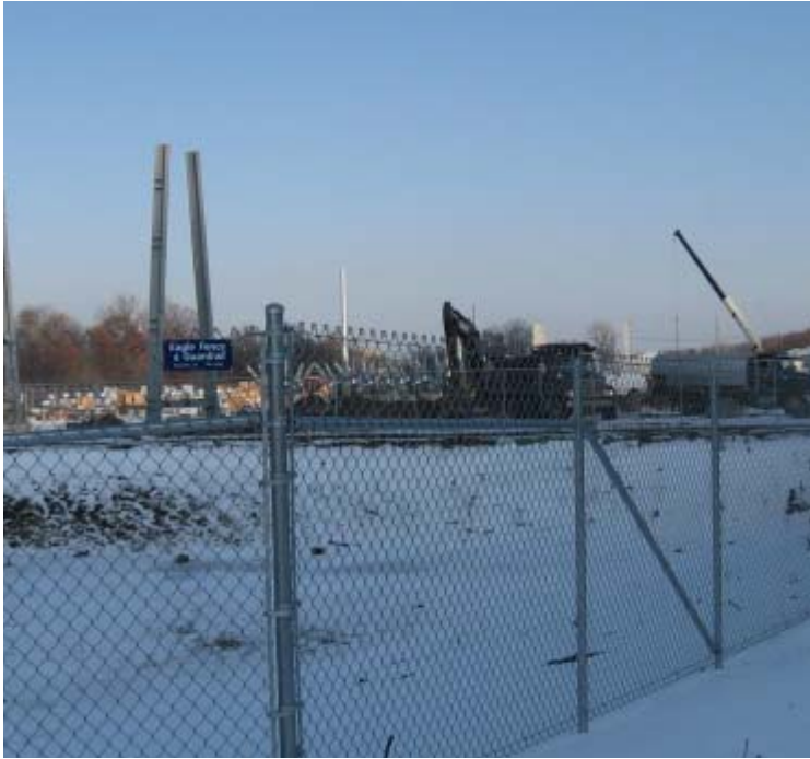
East Devon Substation (Milford): A general view of the construction at the substation.
