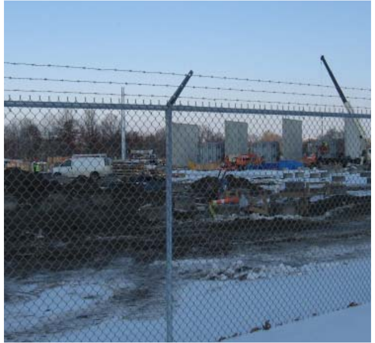
East Devon Substation: An additional view of the construction at the substation.
