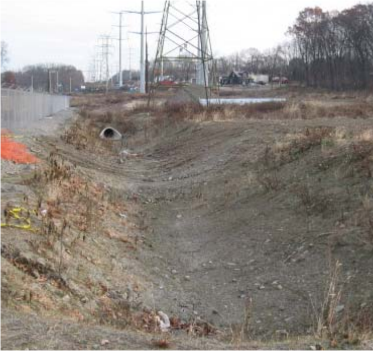
East Devon Substion (Milford): Exposed soils remain in the drainage swale located along the eastern site boundary.
