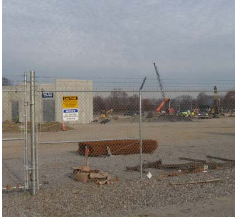
East Devon Substation: A general view of the construction at the substation.
