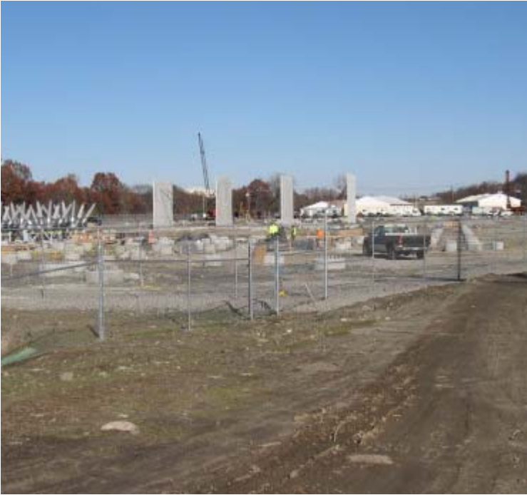
East Devon Substation (Milford): A general view of construction at the substation.
