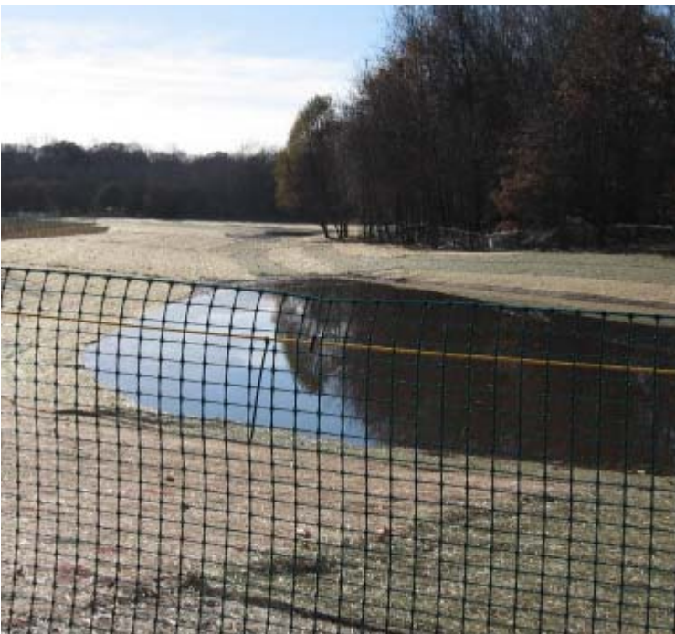
Eisenhower Park (Milford): Erosin blankets have been installed to stabilize soils around the wetland mitigation area.
