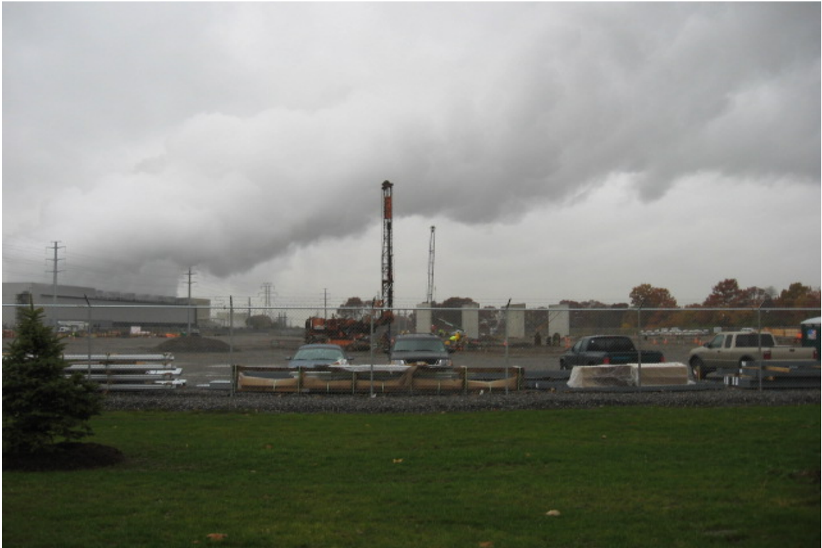
East Devon Subststion (Milford): A general view of construction at the substation.
