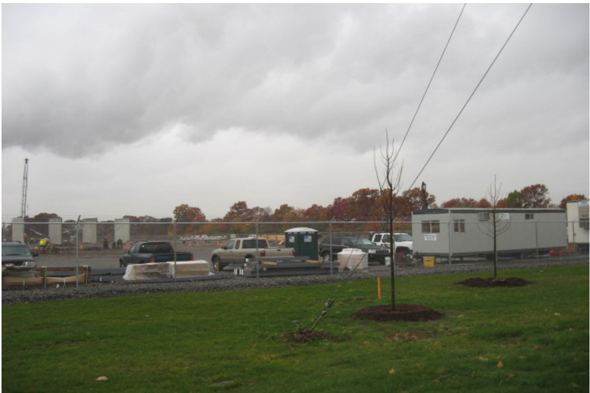
East Devon Substation: An additional view of the construction at the substation.
