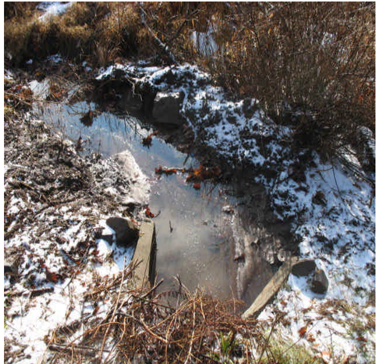
The small channel appears to have widened, possibly from snow melt combined with stormwater. Attention is still needed in this area. When crews return from break, they should remove the sediment prior to the next storm or frozen conditions.
