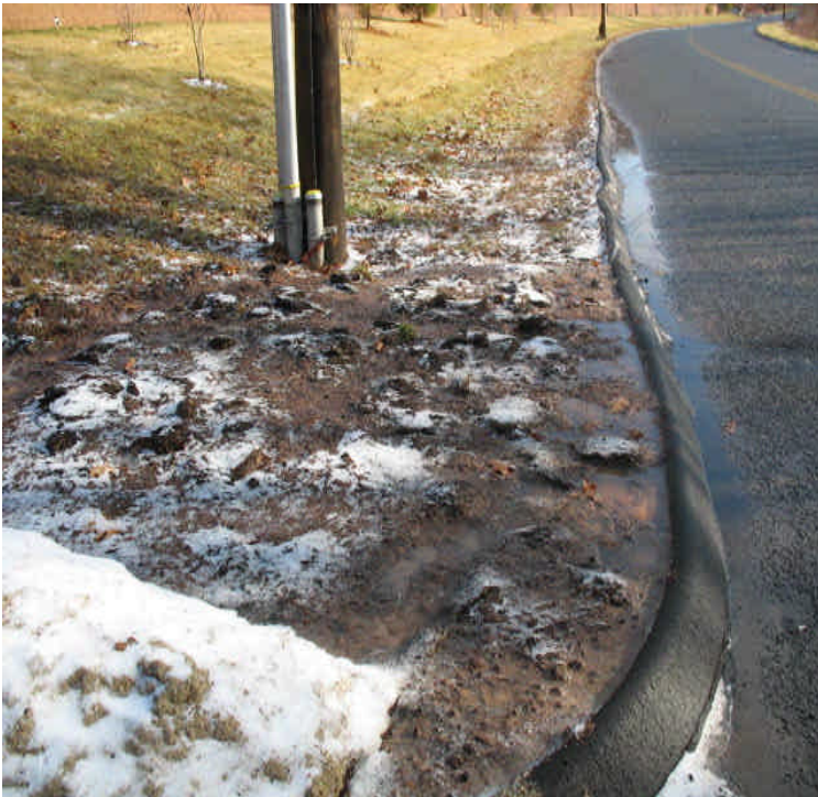
A small disturbed area was noted at the western access curb, likely as a result of plowing.
