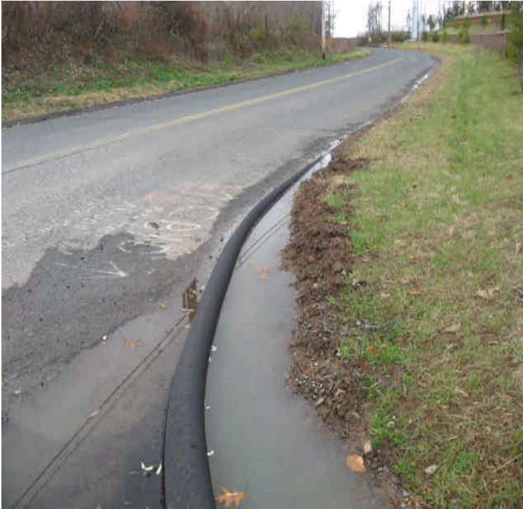
Eastern side of the site, view along Carpenter Lane. New curbing has been installed and turbid run-off from the site is now pooling here and settling before reaching the roadway.
