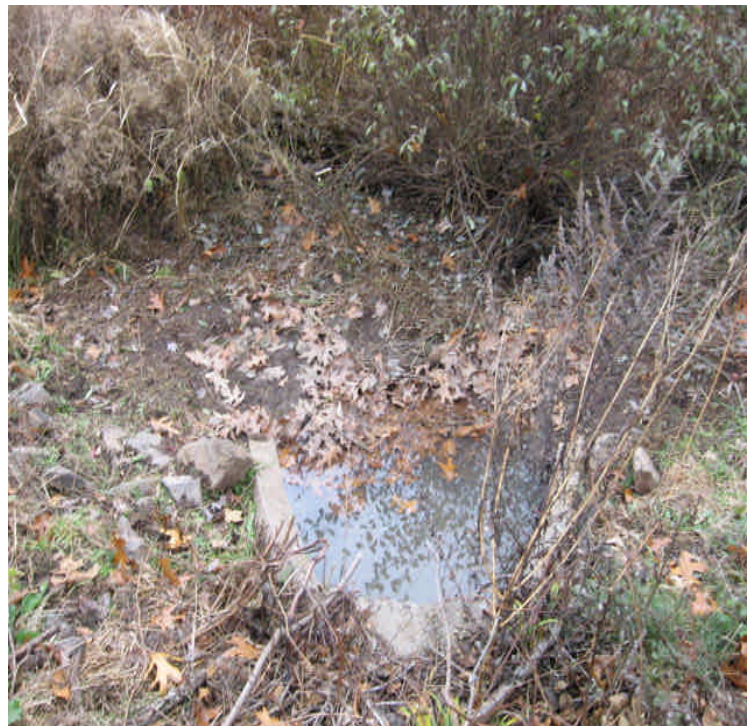
View of the outlet across Carpenter Lane where slightly turbid water was noted in the wetlands following a small rain event. Efforts should be made to remove all visible, settled sediment at the outlet and within the pipe. Seed the disturbed area with wetland mix.
