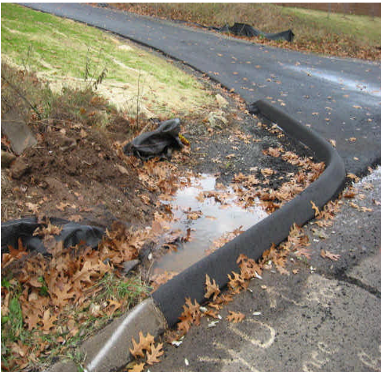
View of the western site access drive which also has newly installed curbing. Clear run-off was noted pooling here.
