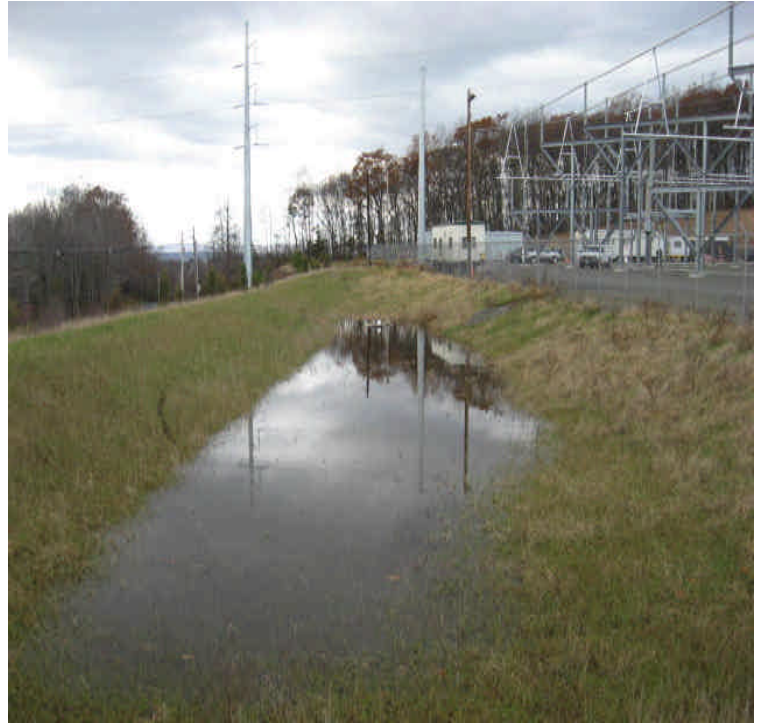
Clear standing water noted at the drain inlets within the detention basin.
