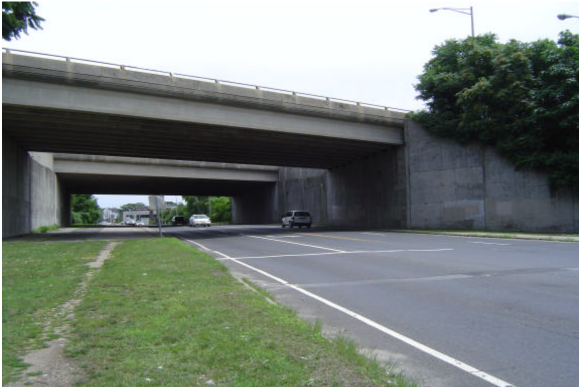
Photo 2: Route 123 (New Canaan Avenue) at the Route 7 Exit 2 Interchange southbound off-ramp looking eastbound at the Route 7 overpasses.
