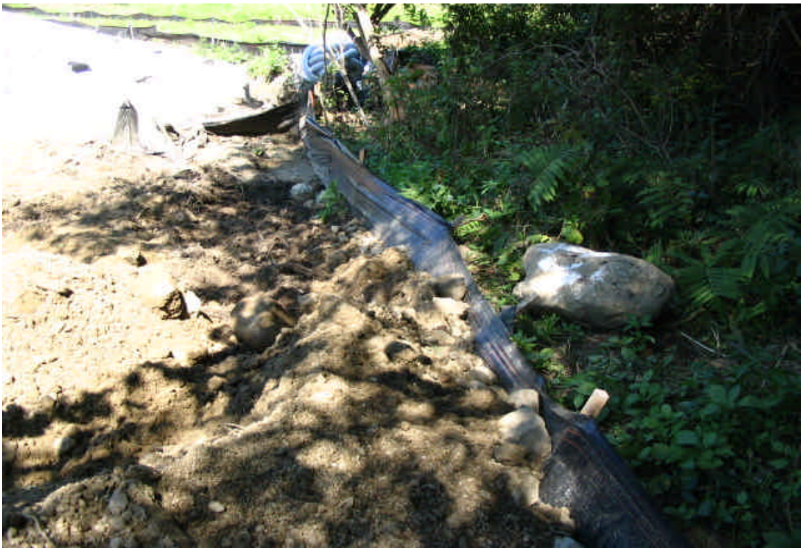
One spot along the silt fence showed some strain due to a soil pile placed too close. The soil will be pulled back and the stakes up-righted. All other controls are in good shape. (9/7/05)
