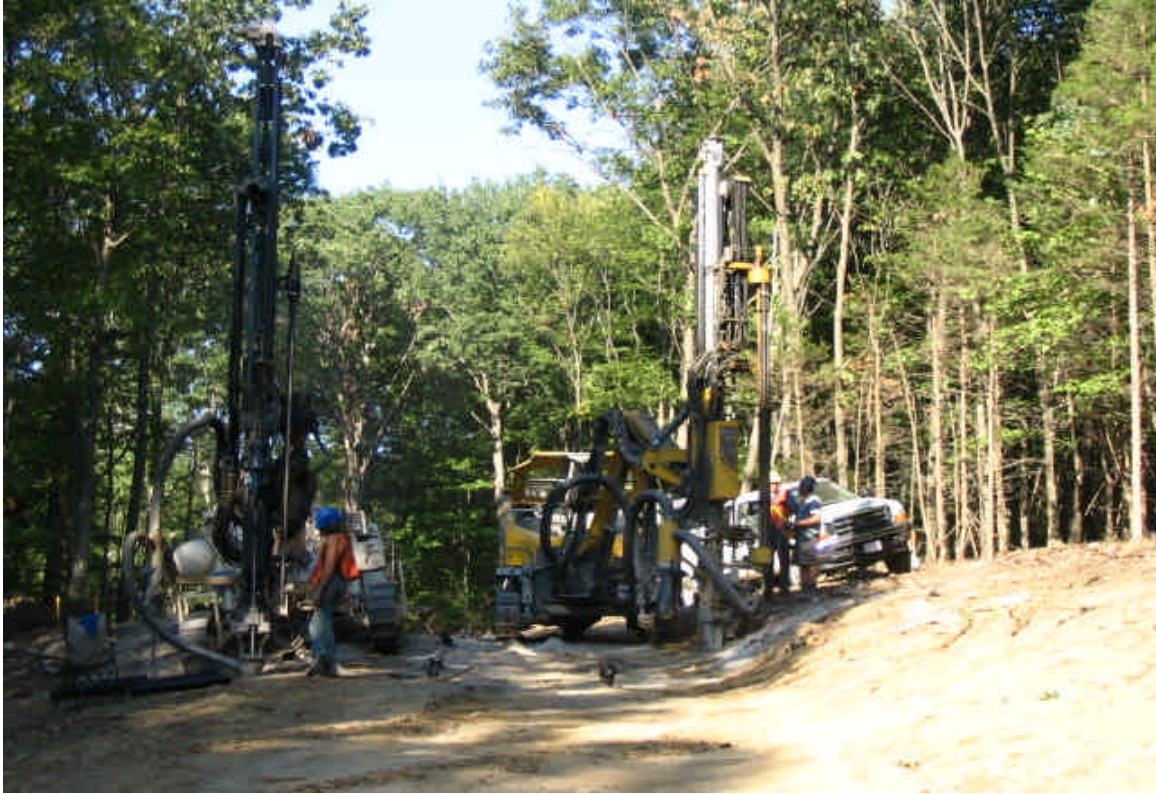
Archers Lane Transition Station: View of the drilling operations in preparation for blasting along the access. Blasting has now occurred in the site. (9/7/05)
