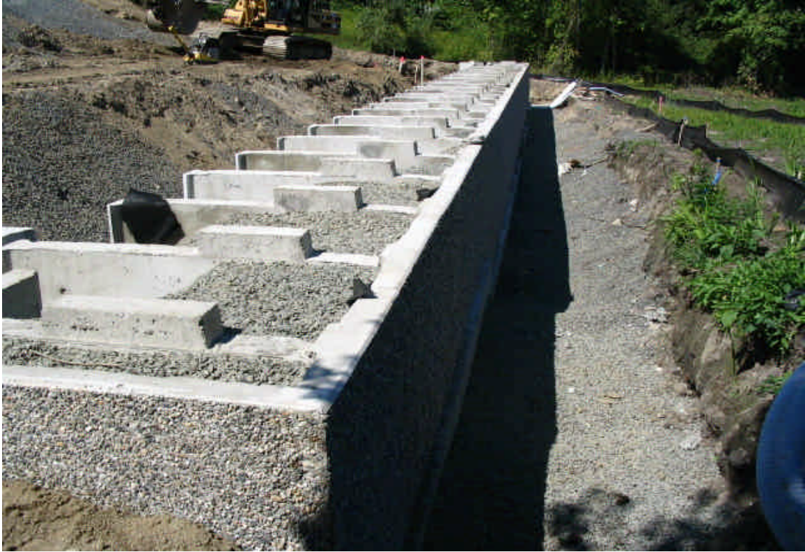
Hoyts Hill Transition Station: Construction continues on the station yard walls and surrounding infrastructure. (9/7/05)
