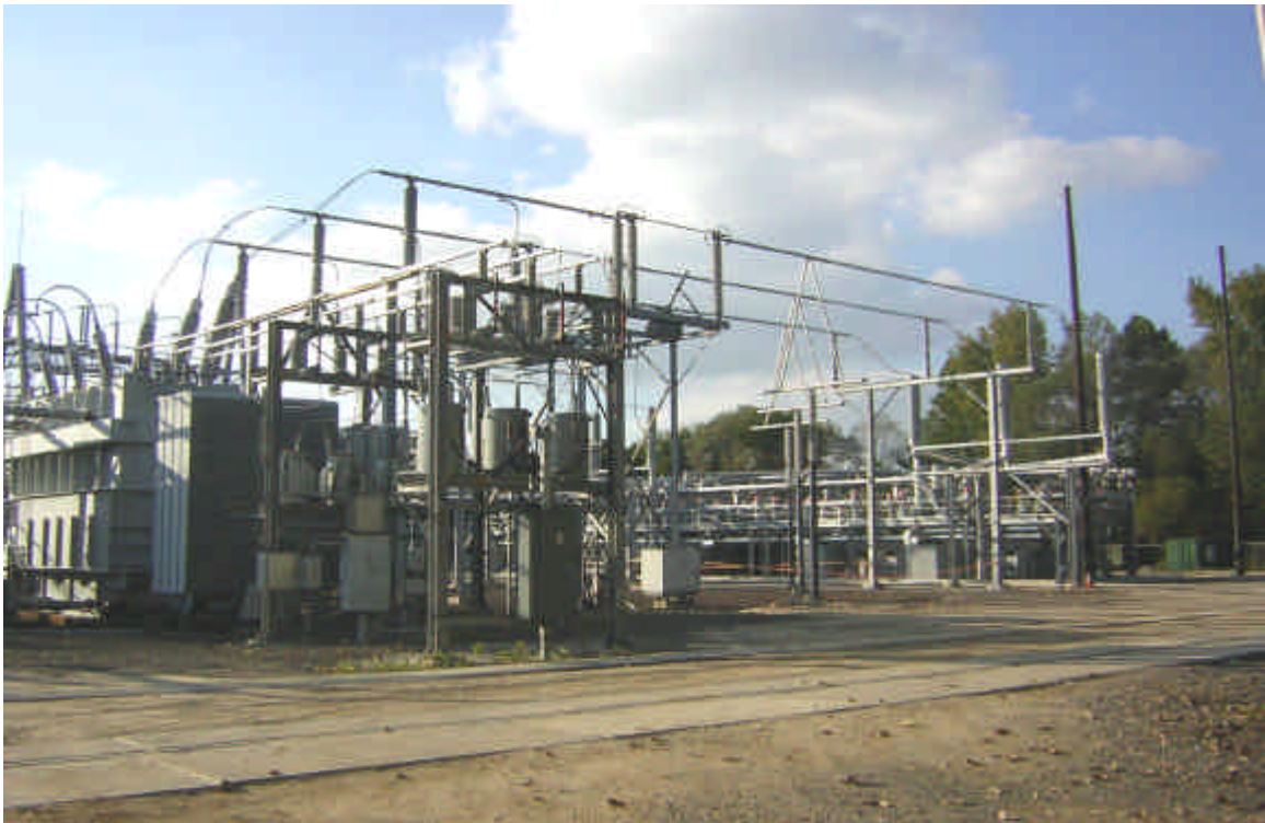
Plumtree Substation: Work continues on structures connecting to the equipment on the concrete pad. 10/5/05
