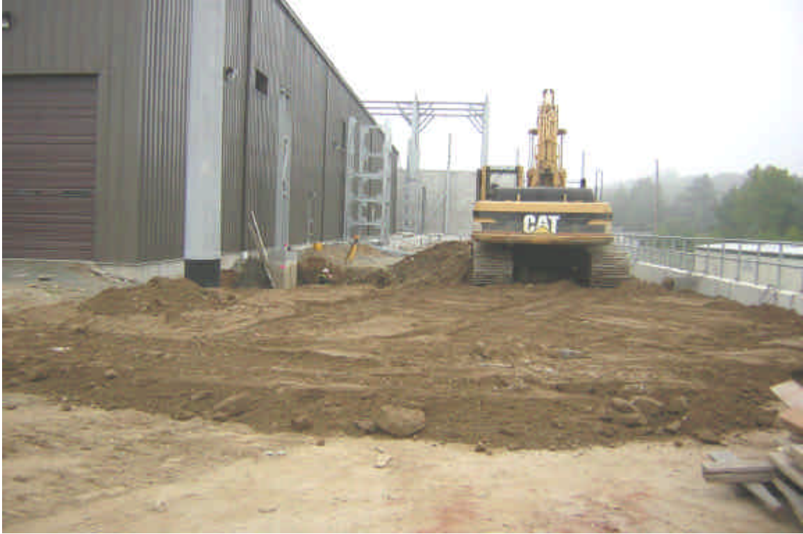
Trenching for the Gas Insulated Transmission Line was occurring on the western side of the GIS building. 10/5/05
