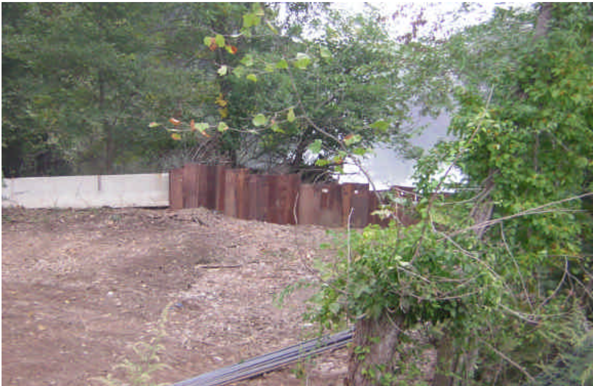
A view of the sheet piling installed as a temporary, partial cofferdam at the northern portion of the temporary work area. 10/5/05
