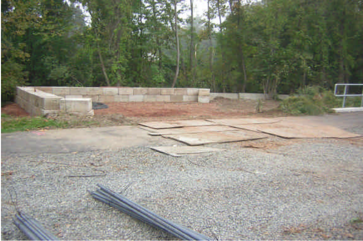
Norwalk Substation: View of the temporary, approved fill placed in the natural overflow area to create a work area and temporary access to the 345kV Turning Structure. 10/5/05
