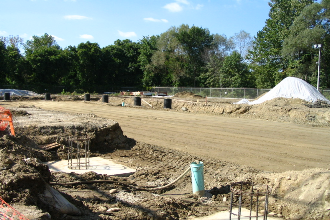
Plumtree Substation: View of the excavation for the GIS concrete pad. The rain had caused delays and problems within the forms and excavations but did not affect areas outside the yard. 9/23/04
