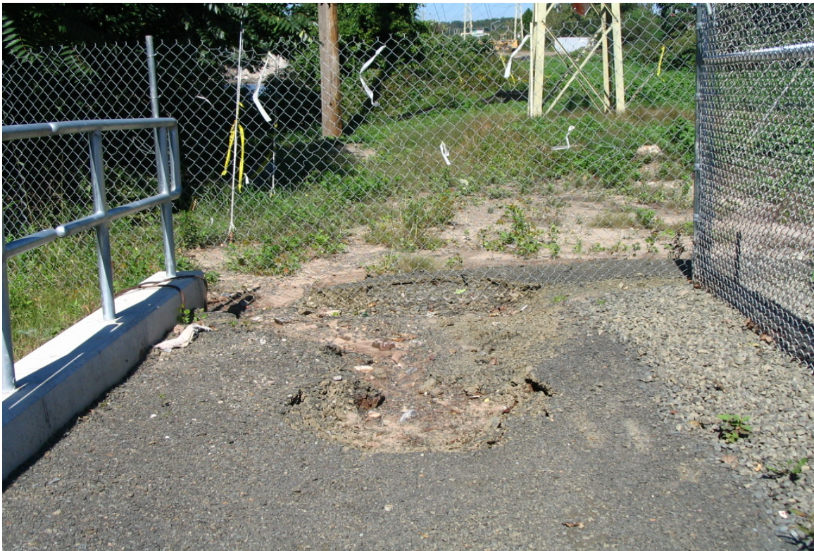
The erosion at the end of the bike path appears to be getting worse and encroaching into the yard. No resource areas are affected and the area will be paved in the coming week. 9/23/04
