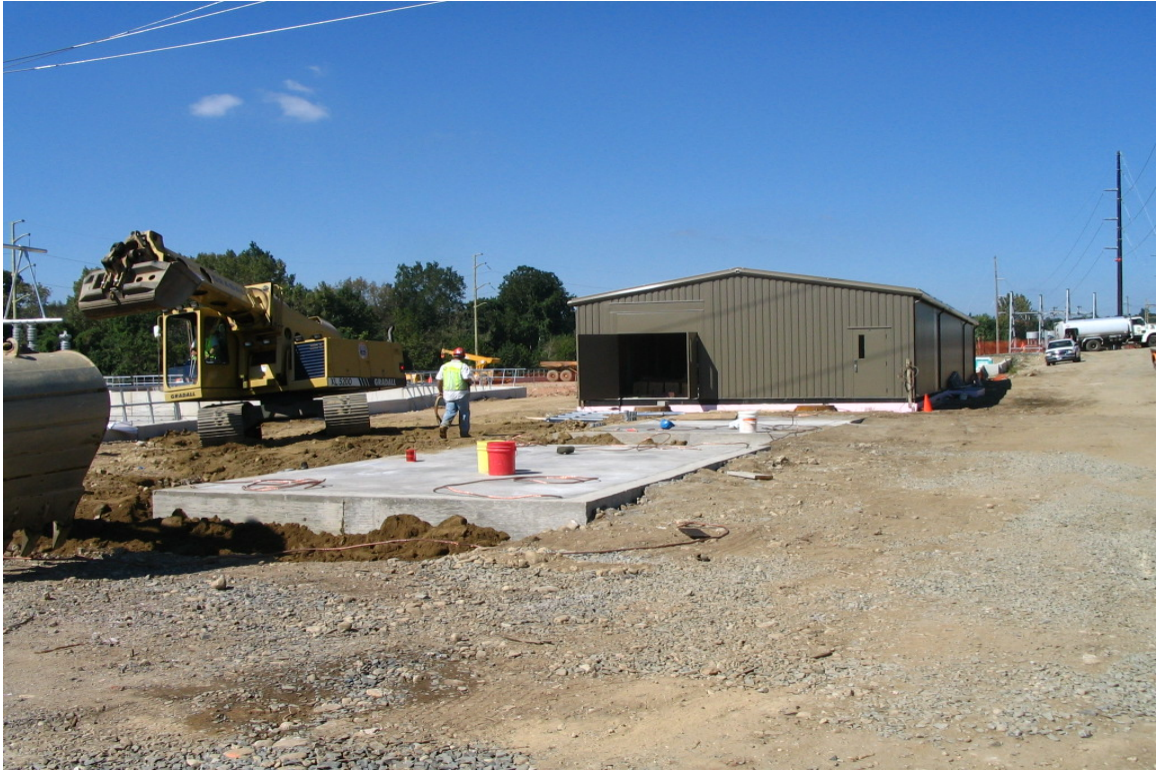
The control house is nearing completion and the conduit bank has been encased in concrete. The stockpiles in the area have been backfilled into the trench. 9/23/04
