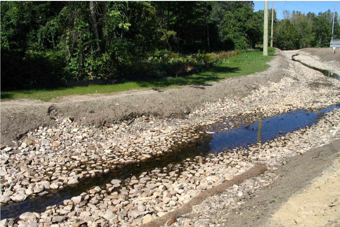
View of the channel with the visible erosion. It is a priority to get vegetation to establish here. Straw mulch should be placed over the seed. 9/23/04
