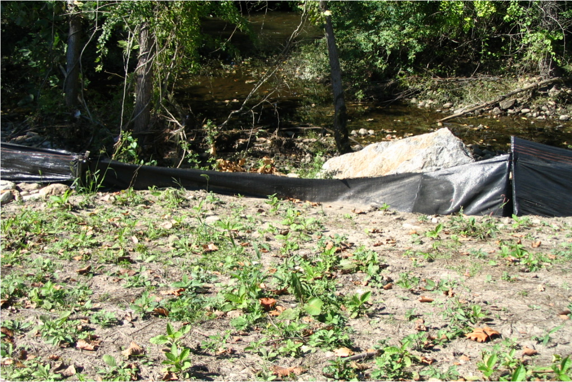
View of a spot near retaining wall where the silt fence could use reinforcement/repair due to strain from sedimentation. 9/23/04
