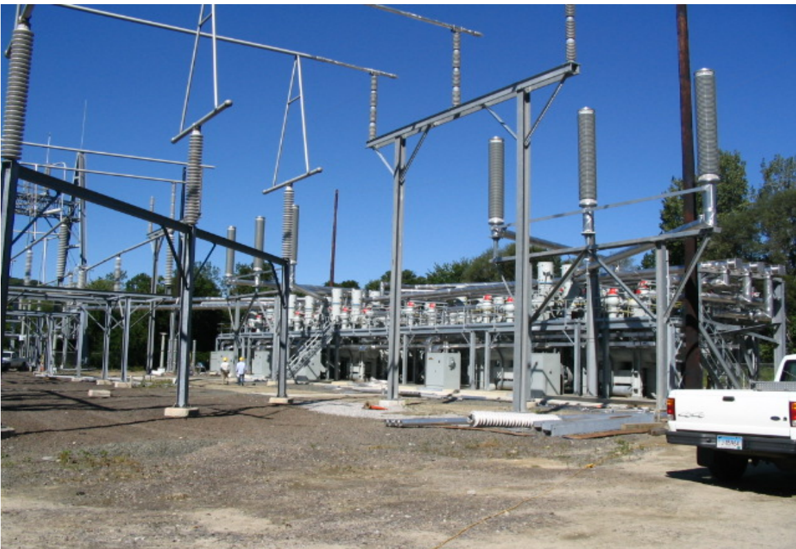
Plumtree Substation: Work continues on structures connecting to the equipment on the concrete pad. (9/21/05)
