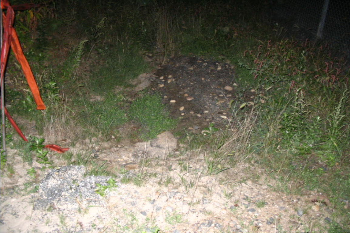
The access road off the Rt. 7 ramp is leading to some sedimentation to the perimeter swale but it remains contained on site and the drive will be paved eventually. (9/21/05)
