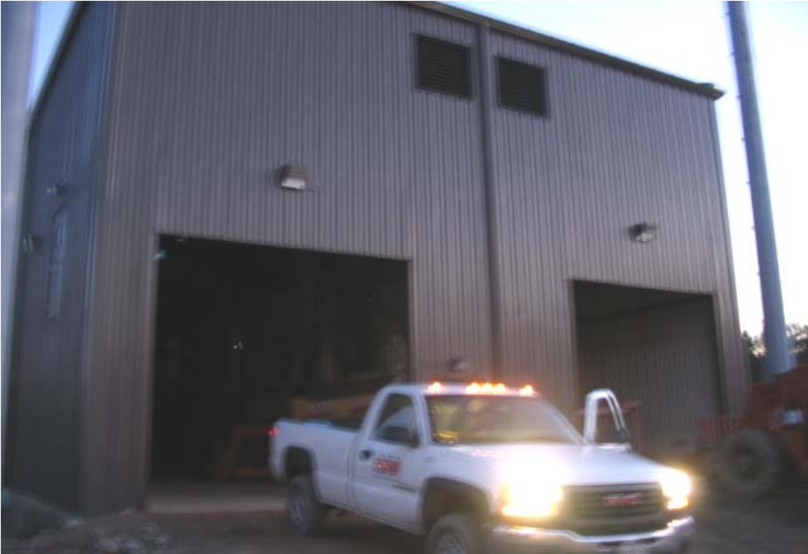
View of the back of the GIS building where installation of equipment is ongoing. (9/21/05)
