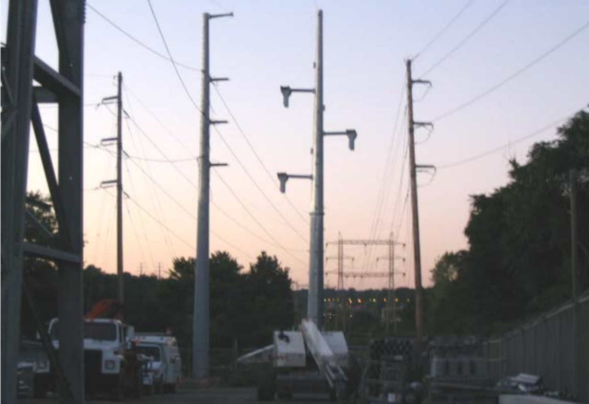
Norwalk Substation: View of the newly installed/constructed 986 and 987 structures at the edge of the ROW at the northern end of the substation. (9/21/05)
