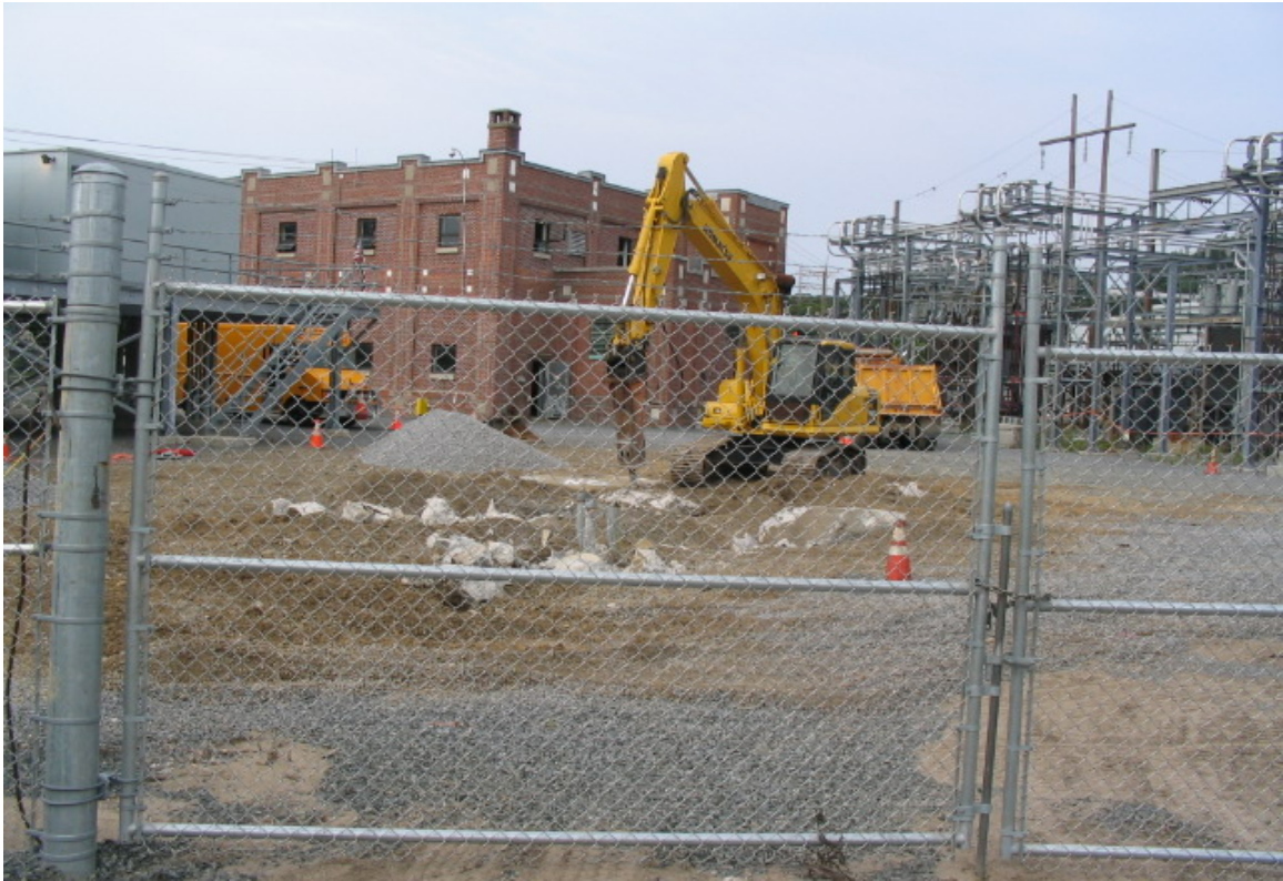
Norwalk Substation: Excavation and breaking up and removal of concrete continues within the live yard. (8/19/05)
