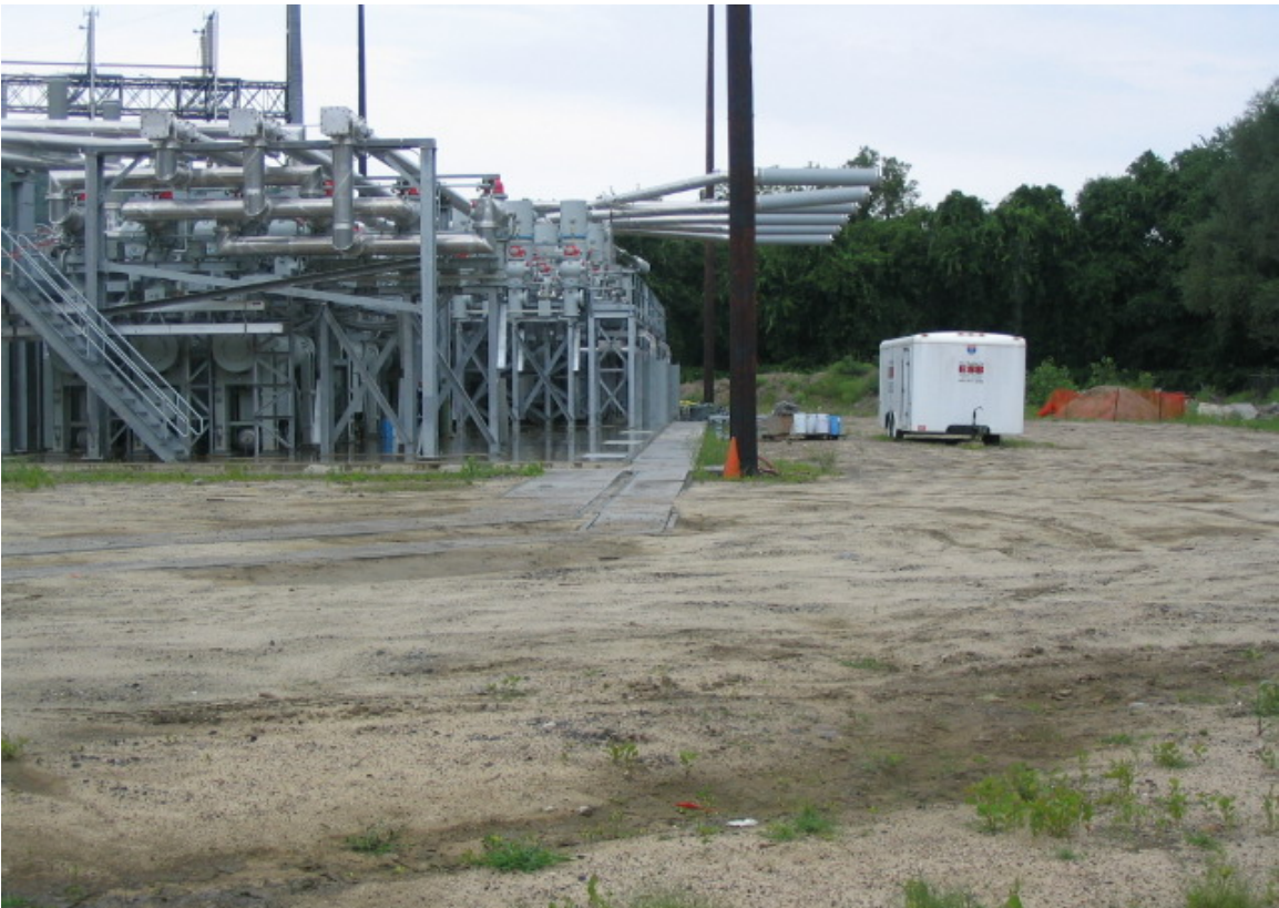
Plumtree Substation: General view of the site. No soil disturbing activities have been occurring. (8/19/05)
