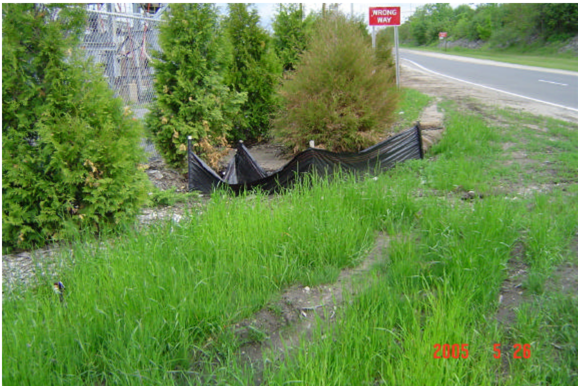
Vegetation is returning around the inlet however, erosion at the base of the silt fence is still occurring. (5/26/05)
