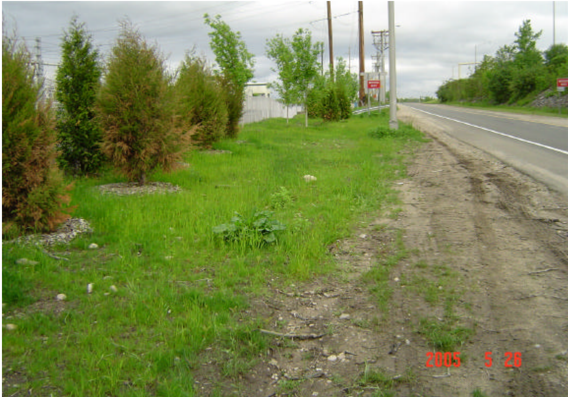
Vegetation is returning along the Rt. 7 ramp and within the earthen swale. (5/26/05)
