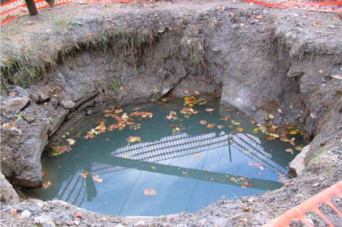
The excavation was filled with water following the rain but sediment had settled out. Dewatering will have to occur to a corral since the wetlands are located adjacent. (10/19/05)
