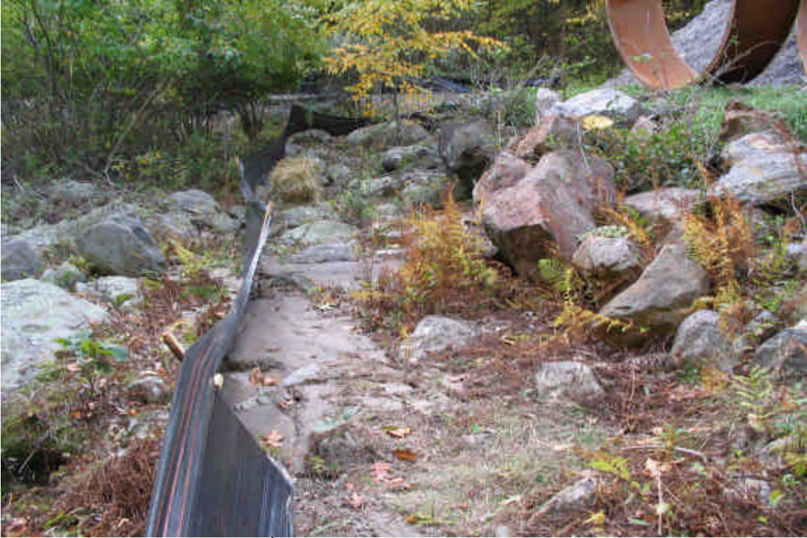
Overhead ROW: View of the 2 nd structure in from Gallows Hill. Some sediment ran off from the stockpile and accumulated at the silt fence. Some also filtered through the rock to the wetland. Haybales will be added here to help prevent this and sediment will be hand removed. (10/19/05)
