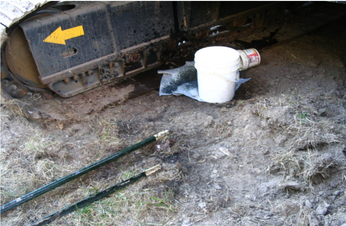
View of the hydraulic leak being contained with the bucket and pads for the time being. Mechanics were on site and the affected soil will be shoveled up and removed. (10/5/05)
