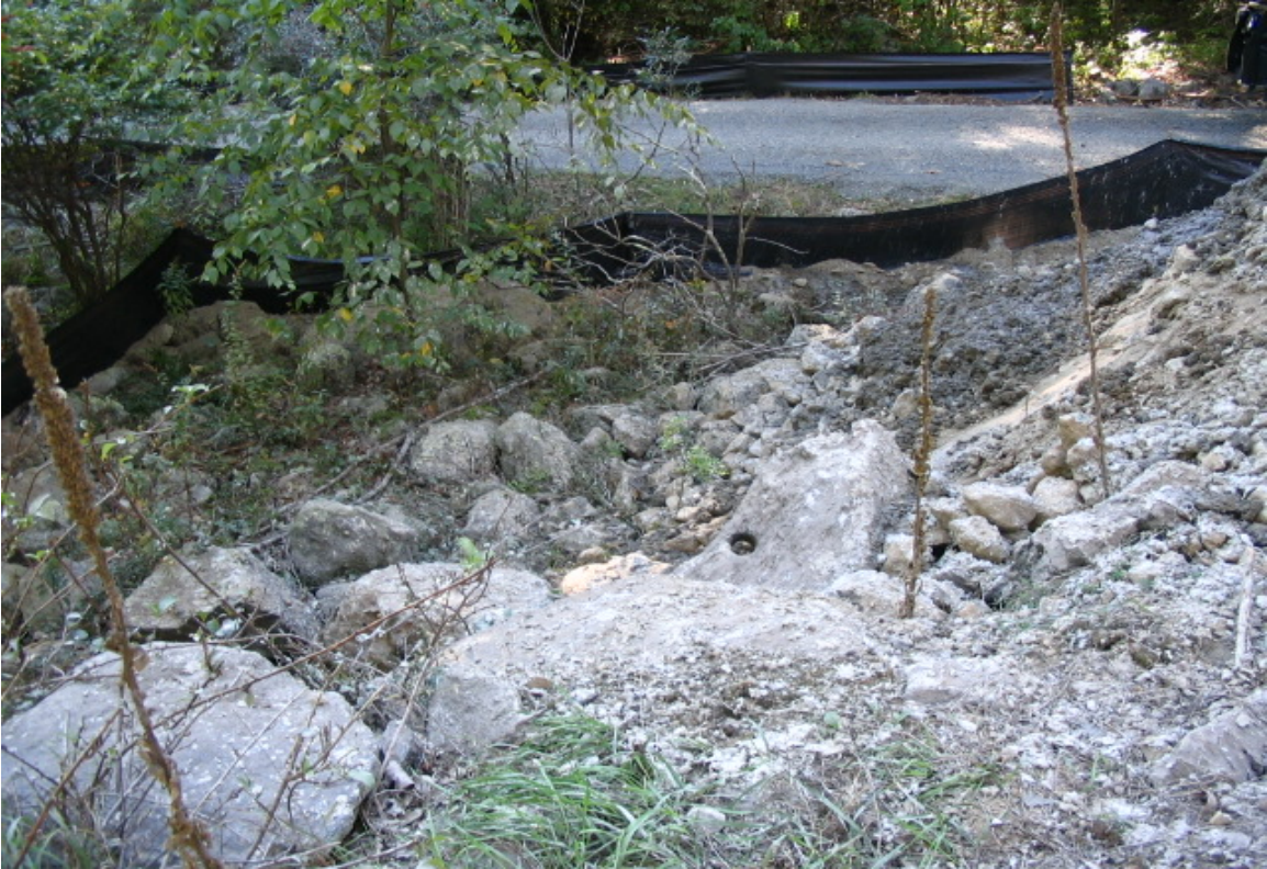
The pile of excavate from the structure foundation hole is immediately adjacent to the silt fence. Continue to maintain this fence well until this stockpile can be removed. Staked haybales would be a good addition here. (10/5/05)
