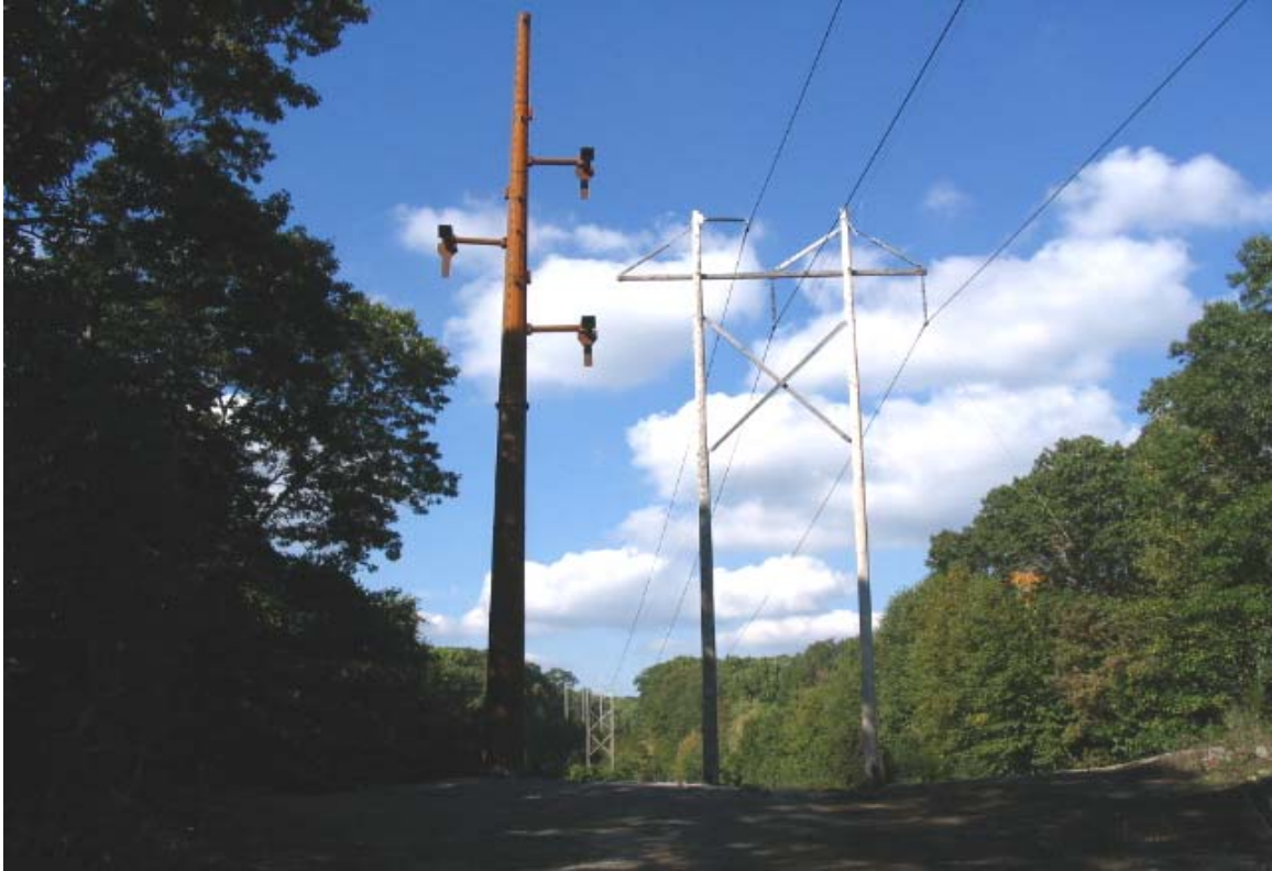
Overhead ROW: View of the riser structure recently installed just off Gallows Hill Rd. (10/5/05)
