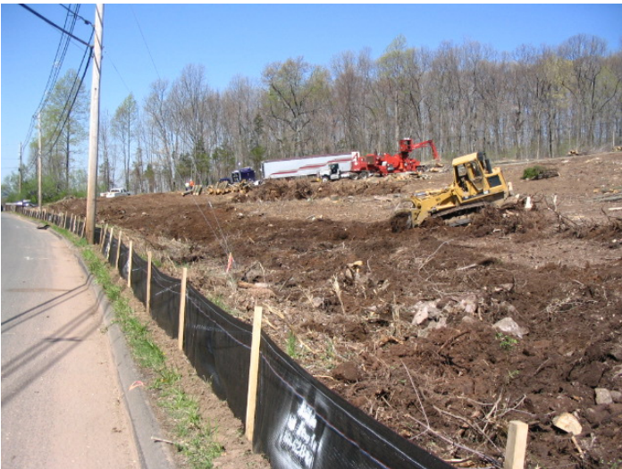
Clearing and grubbing, wood chipping visible in rear, viewed looking toward west-northwest along Carpenter Lane
