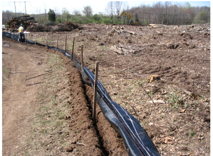
Clearing, grubbing south side of site, viewed toward east. Silt fence is being installed at this time.
