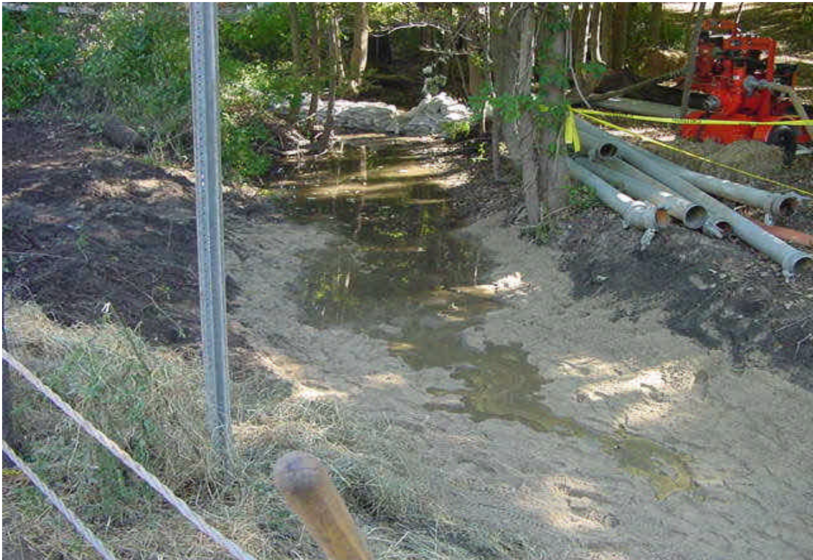
115kV (Rt. 58 Stream Cut) The stream cut at Sara's Way has been completed and restoration of the area was in progress. Water was just beginning to be released to the stream channel. (9/29/05)
