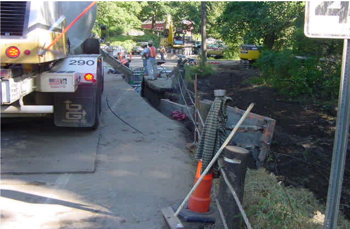
View of the trench work returning to the roadways adjacent to the stream cut. (9/29/05)
