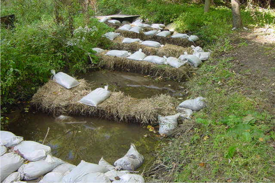
View downstream of the work. A number of check dams were placed to filter the stream flow. (9/29/05)
