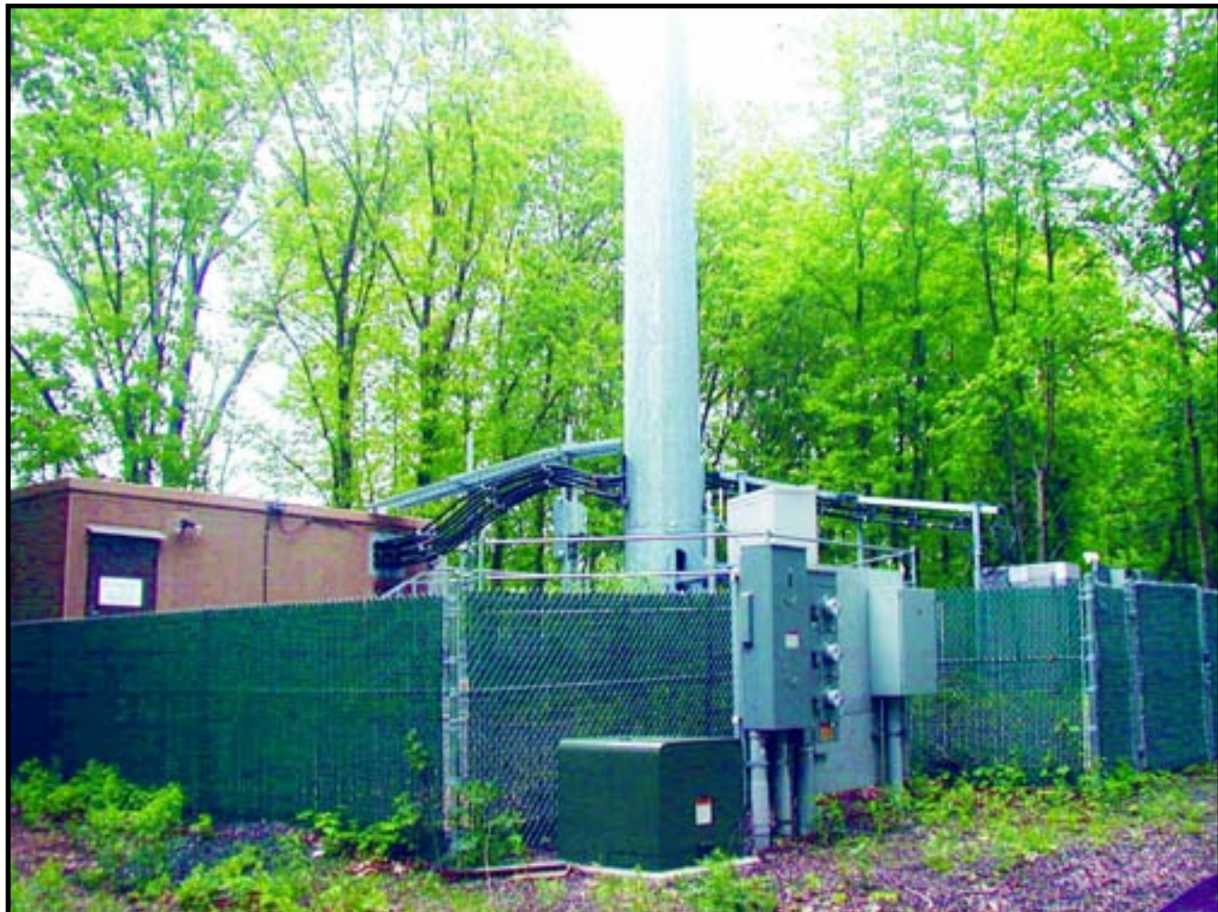
Figure-65. 300 Governor's Highway in South Windsor, CT. Photograph taken in May of 2004.
