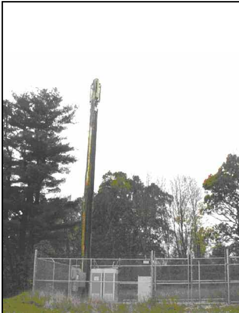
Figure-27. A 55-foot wooden pole located at 111 Middle Turnpike in Mansfield, CT (also known as a “brown stick”). Photographed in October of 2004.
