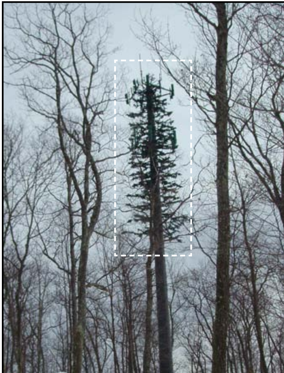
Figure-24. A 110-foot telecommunications facility disguised as a tree located at 70 Herb Road in Sharon, CT. Photographed in February of 2007.
