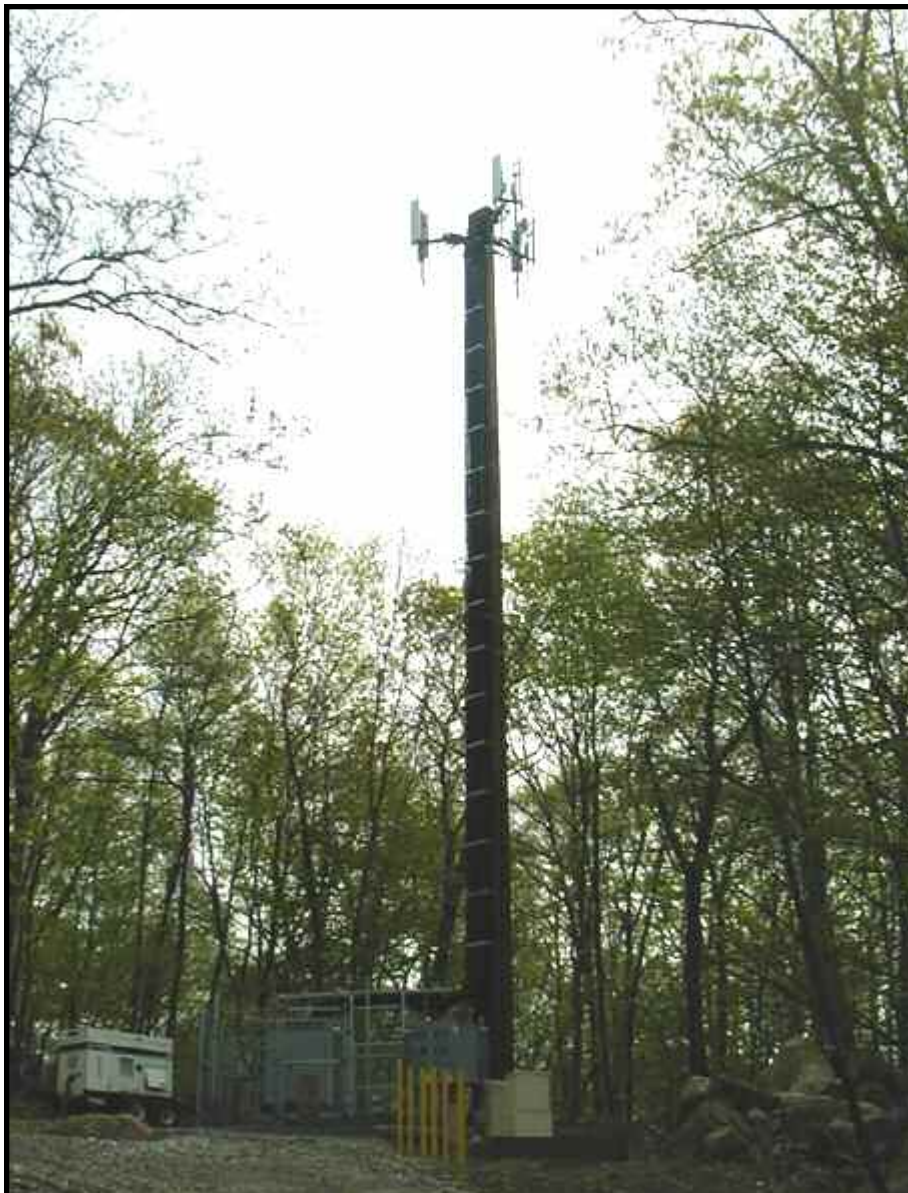
Figure-26. An 80-foot wood laminate pole located at 41 Padanaram Road in Danbury, CT. Photographed in May of 2006.
