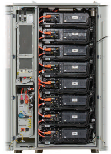
Battery cabinet (interior view with 8 battery modules)
