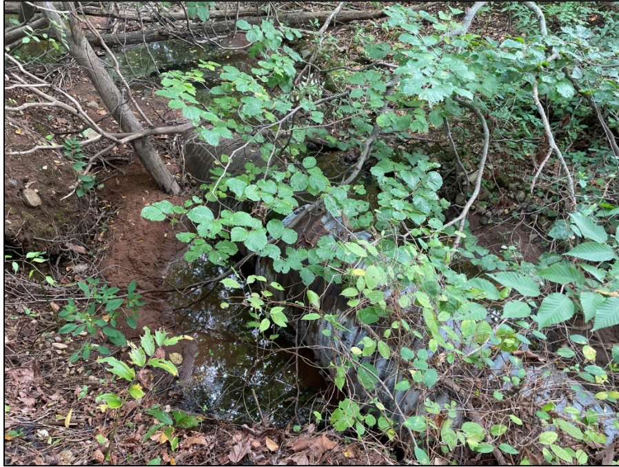
Photo 1: View of eroded culvert at WF-1 and WF-1X looking north.
