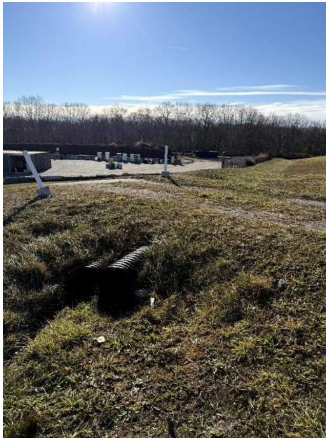
Photo 19: Existing stormwater control features (15" CPP) under existing access road to top of landfill. Picture is looking southwest towards transfer station.
