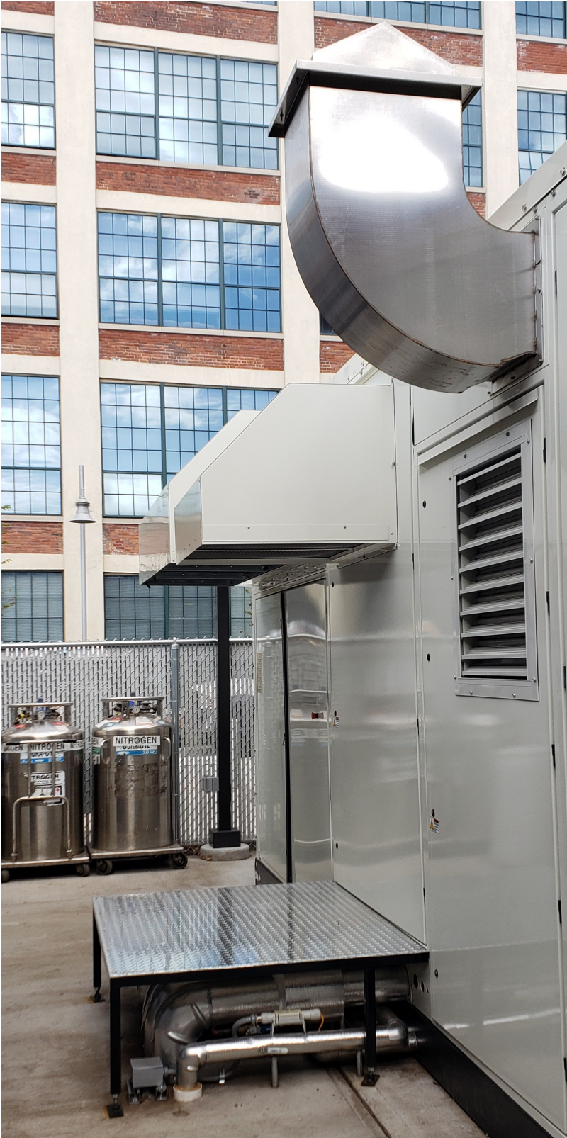
Figure 10. Photo of the Fan Side of the Power Module in Bridgeport 7
