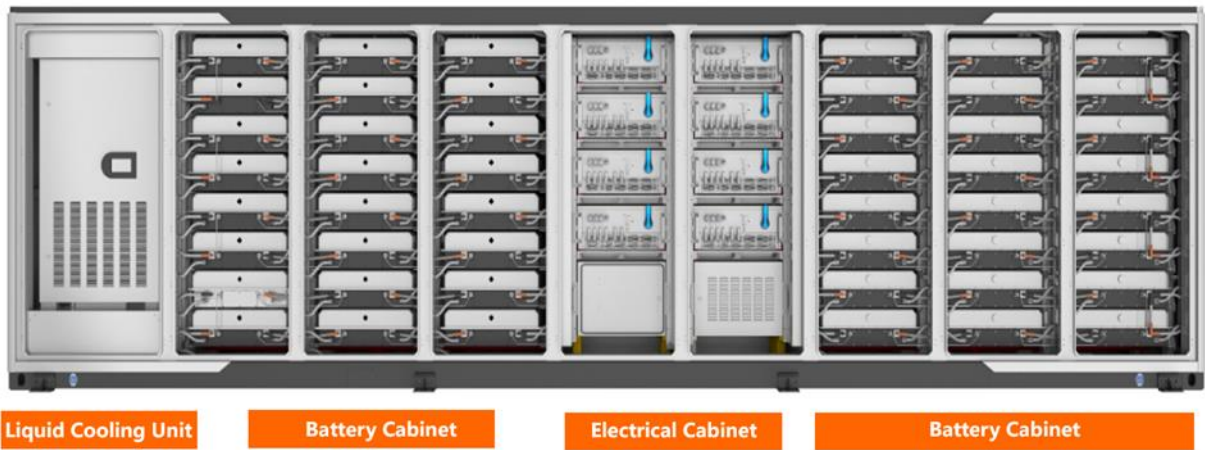
Figure 12: Battery Unit (ST2752UX) - Doors removed to expose internals: Liquid cooling unit, Battery Cabinets and Electrical Cabinet.
