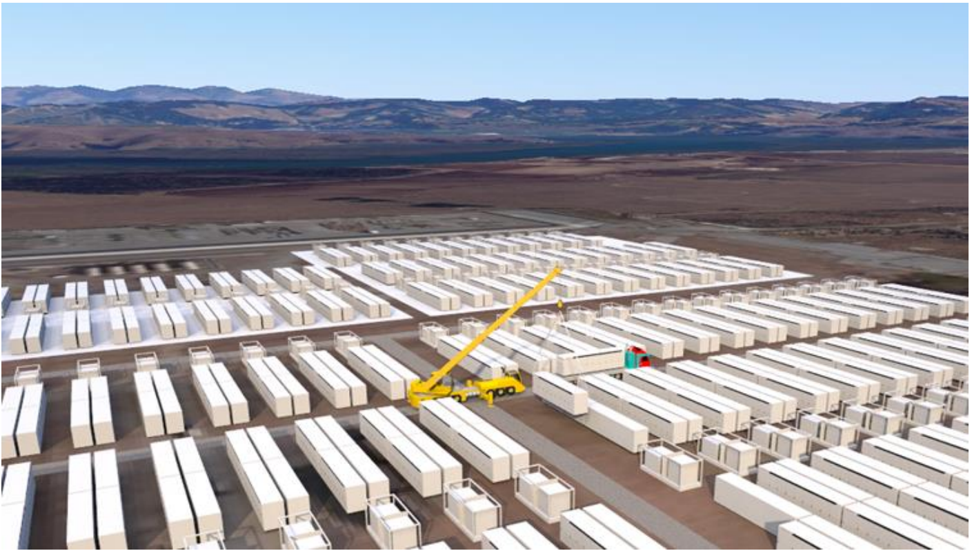
Figure 8: Typical battery site (power plant). Ensure fire hoses and typical spray can reach various areas to manage fires
