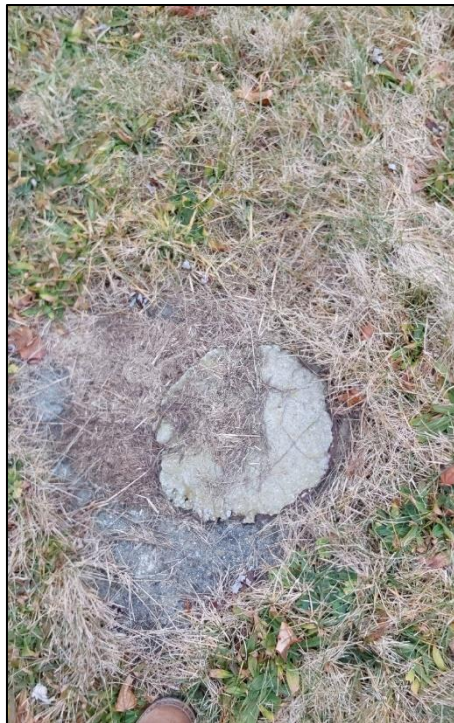
Photo 6. Close up of hole filled in with concrete in the facility area.
