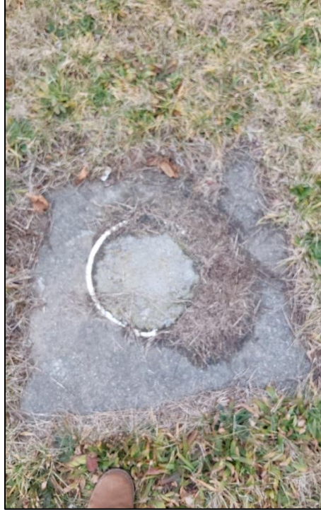
Photo 5. Close up of hole filled in with concrete in the facility area.
