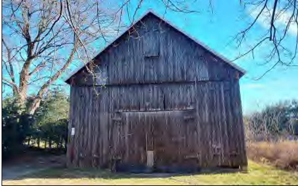
Photo 27. Overview of northwestern elevation of 186 Foster Street (Resource 49). Photo facing to the southeast.
