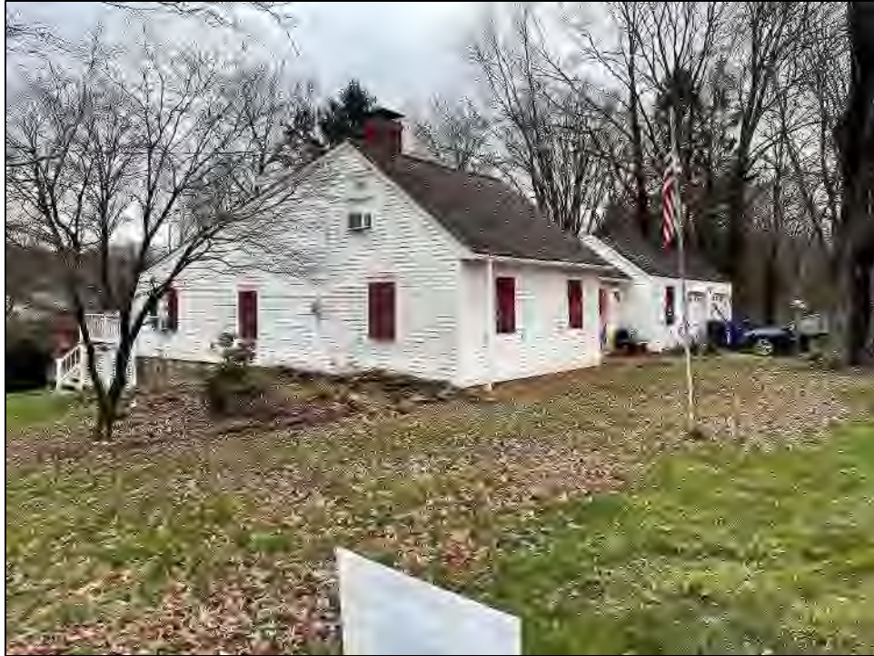
Photo 17. 3/4 view of southwestern elevation of 496 Oakland Road. Photo facing to the northeast.
